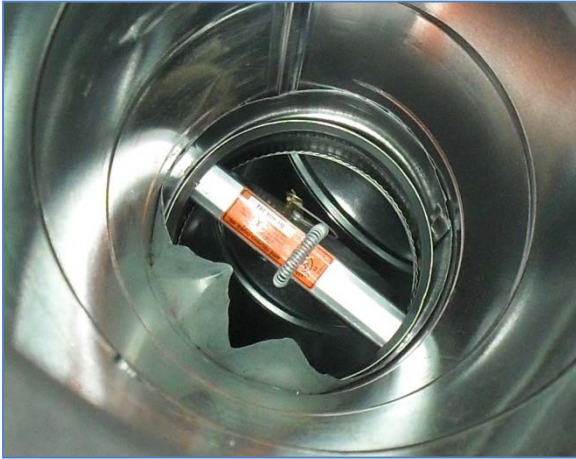
Figure 4.5: Fire Damper and Duct-Connection Restrictions in Outdoor Air Duct
