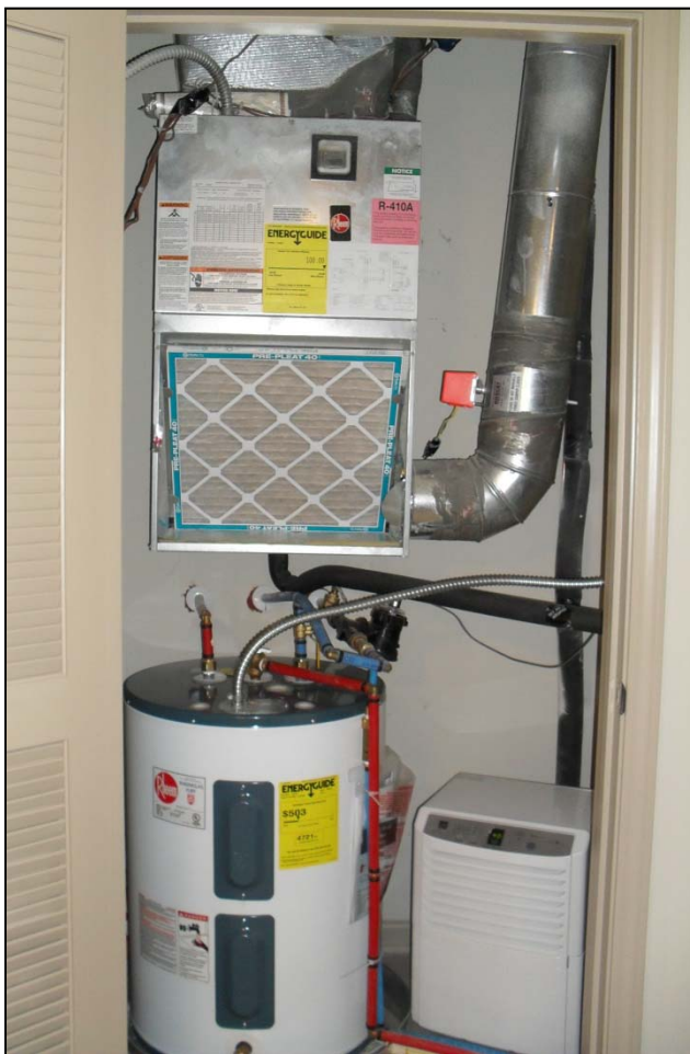
Figure 3.1: Typical Mechanical Closet in Test Building
