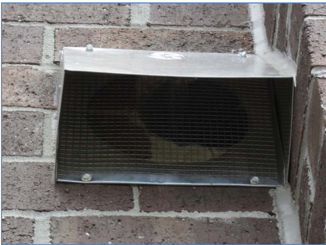
Figure 4.4: Misaligned Wall Cap on Outdoor Air Intake
