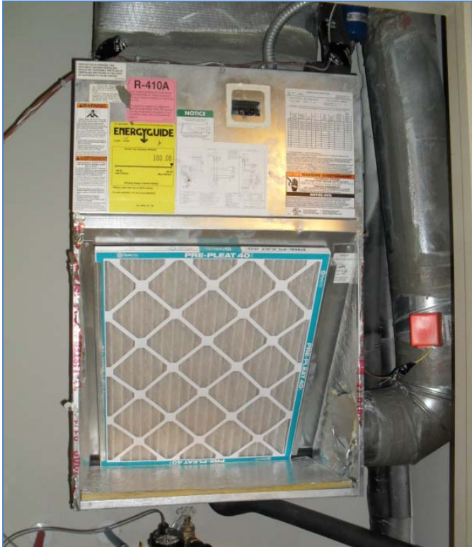
Figure 4.3: Closed Outdoor Air Flow Damper
