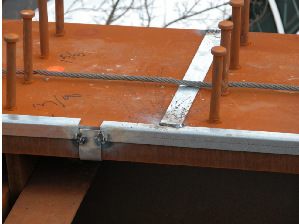
Figure 65: Light-gage metal strap attached to longitudinal light-gage angles on opposite side of fascia girder
