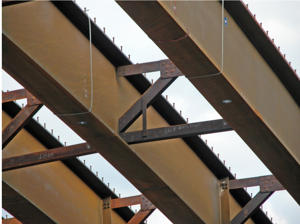
Figure 63: View of the cross frame with missing connection plate
