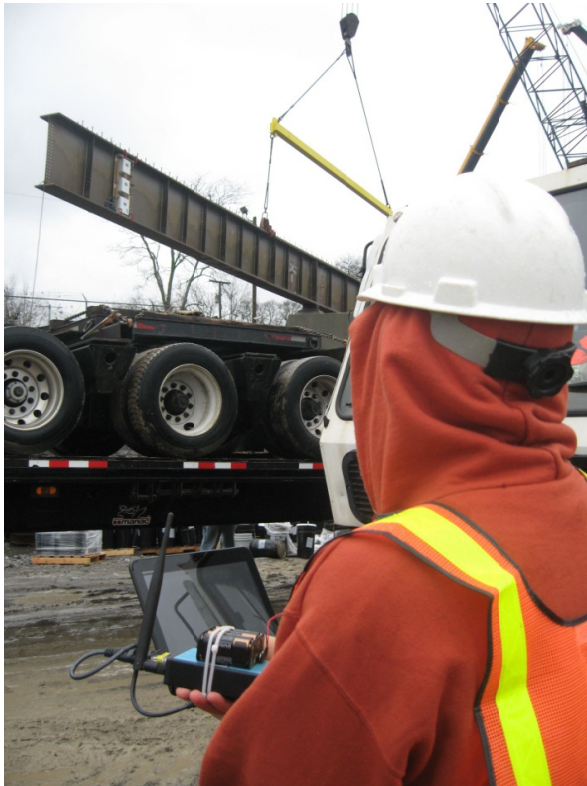
Figure 26: Downloading of data remotely from one of the data acquisition boxes
