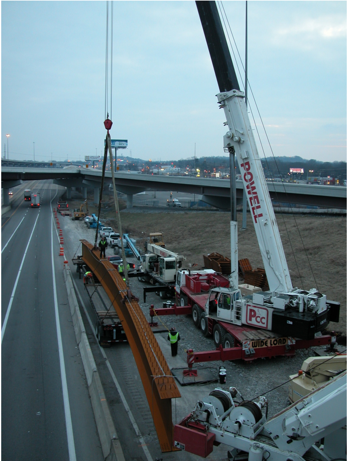
Figure 52: View of the 175-ton lifting crane located on the south side of I-40 just prior to the lifting of girder 131E7 (Photo taken from the Robertson Ave. bridge)
