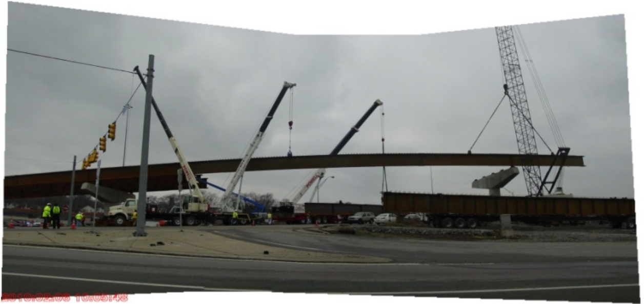
Figure 50: View showing girder 125A5 being stabilized by a holding crane and the lifting crane released to pick girder 124B5
