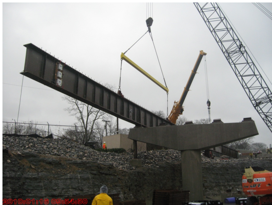
Figure 35: Girders 105A1 and 110A2 located on supports, spliced together, and held by cranes
