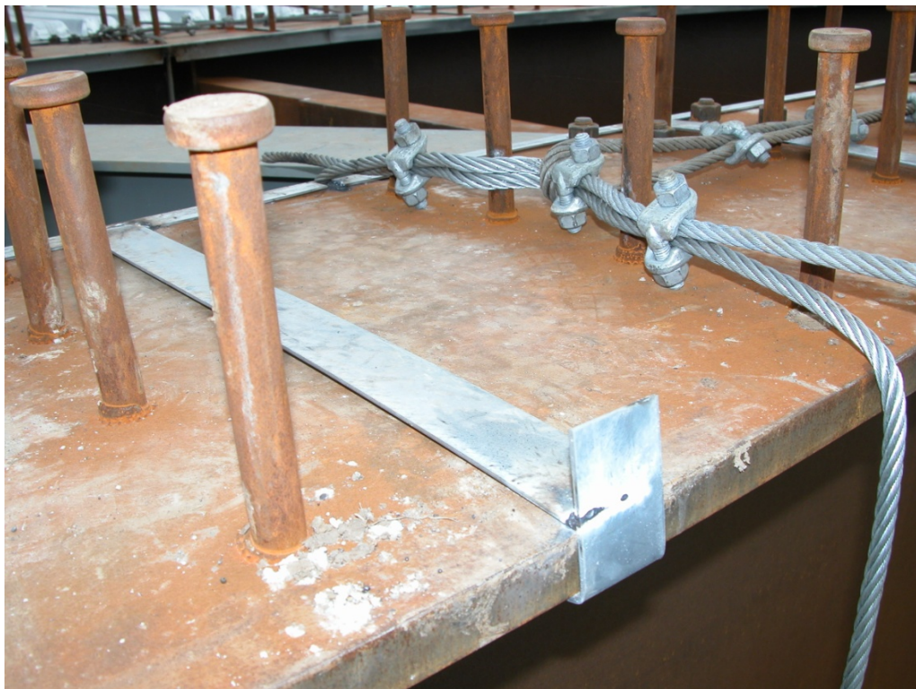
Figure 64: Light gage metal strap attached to the top flange of fascia girder
