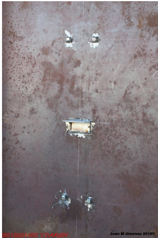
Figure 22: Nuts for two strain gages and support bracket for clinometer have been welded to the girder and are ready for installation of the instrumentation
