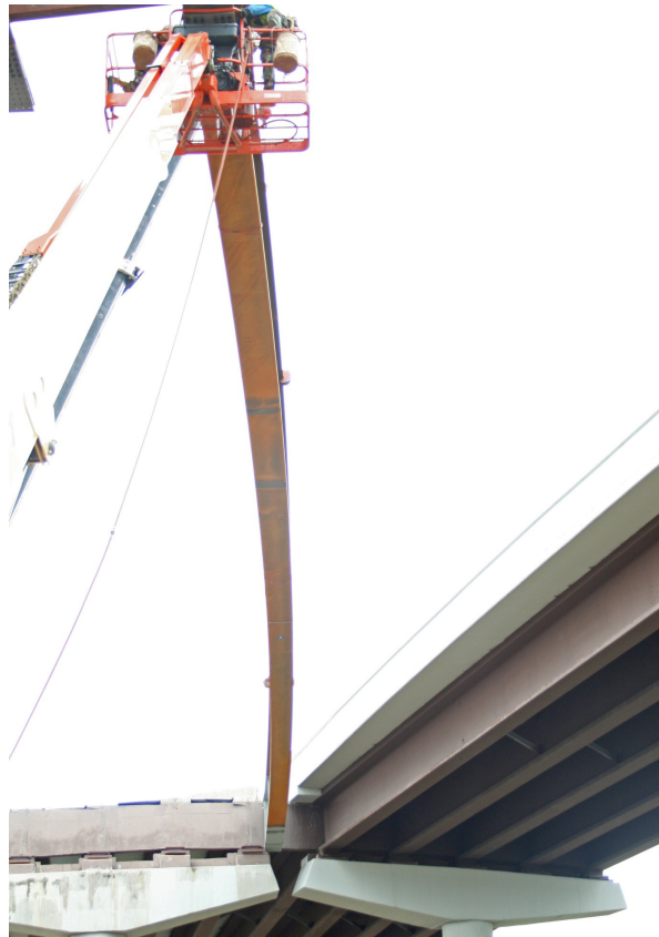
Figure 61: Twisting in Girder 175A15
