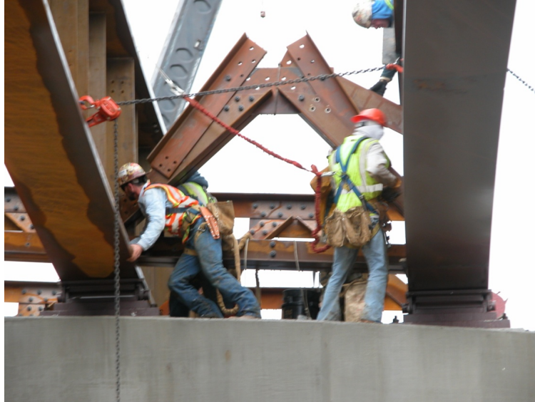
Figure 46: Installation of bearing line cross-frame between girders 119B4 and 118C4 at Bent 1
