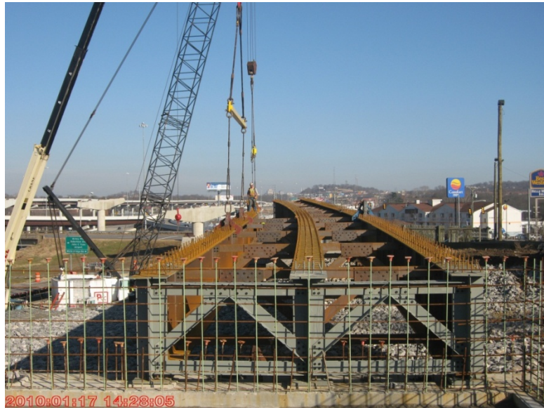
Figure 42: View showing two cranes holding the third girder line while making the splice between 103C1 and 108C2
