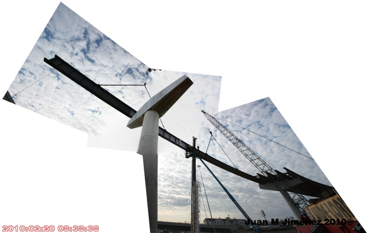
Figure 55: View of Span 5 with girders 145A9 and 150A10 up, with the lifting cranes still engaged, and with the holding crane attached to 145A9
