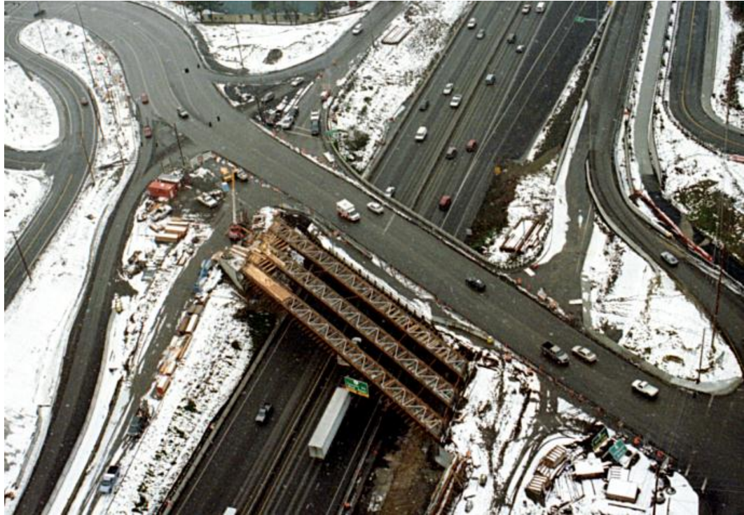
Figure 4.6. ETSSS2, Sylvan Bridge over Sunset Hwy in Multnomah Co., OR. (Courtesy of H. Seradj, ODOT).
