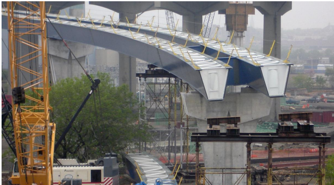
Figure 1.1. Tub-girder bridge under construction at the Marquette Interchange, Milwaukee, WI. (Courtesy of T. Shkurti, HNTB).
