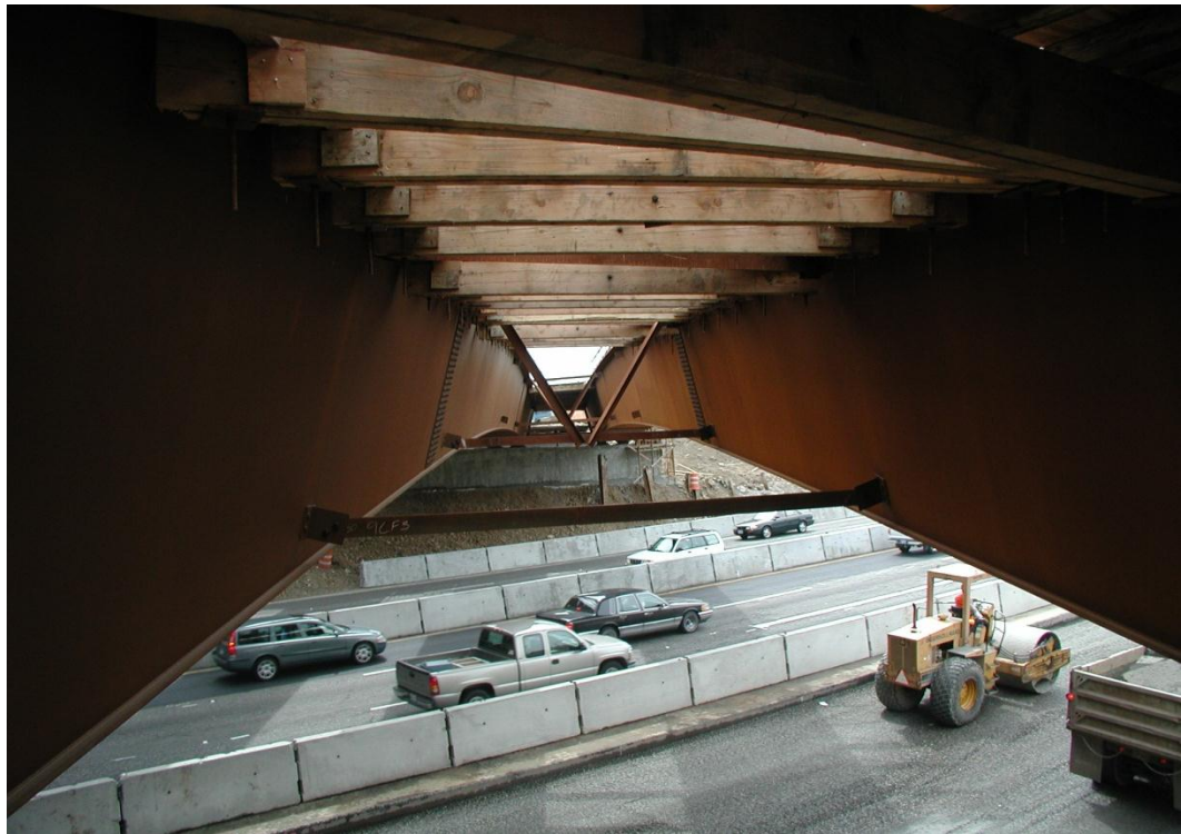
Figure 4.7. ETSSS2, Sylvan Bridge over Sunset Hwy in Multnomah Co., OR. (Courtesy of H. Seradj, ODOT).
