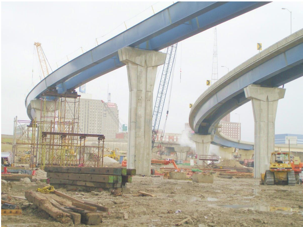
Figure 4.12. ETTTCR 15, Unit B-40-1122 of the Marquette Interchange, Milwaukee, WI. (Courtesy of T. Shkurti, HNTB).
