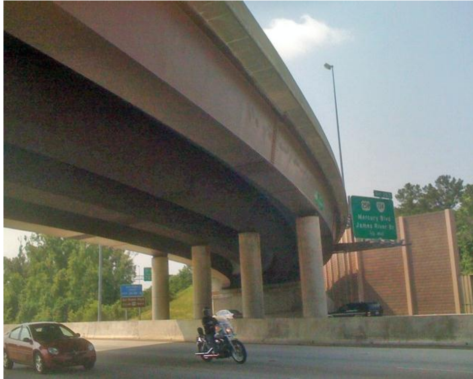
Figure 4.15. ETCCS6, Magruder Blvd. bridge over I-64 in Hampton, VA. (Courtesy of D. White).
