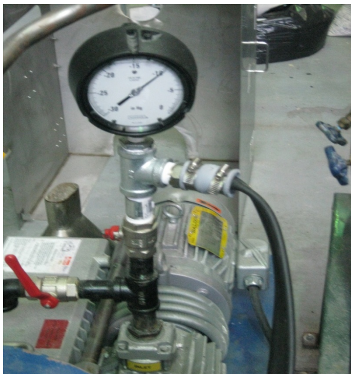
Figure 3.6: Vacuum pump with a gauge
