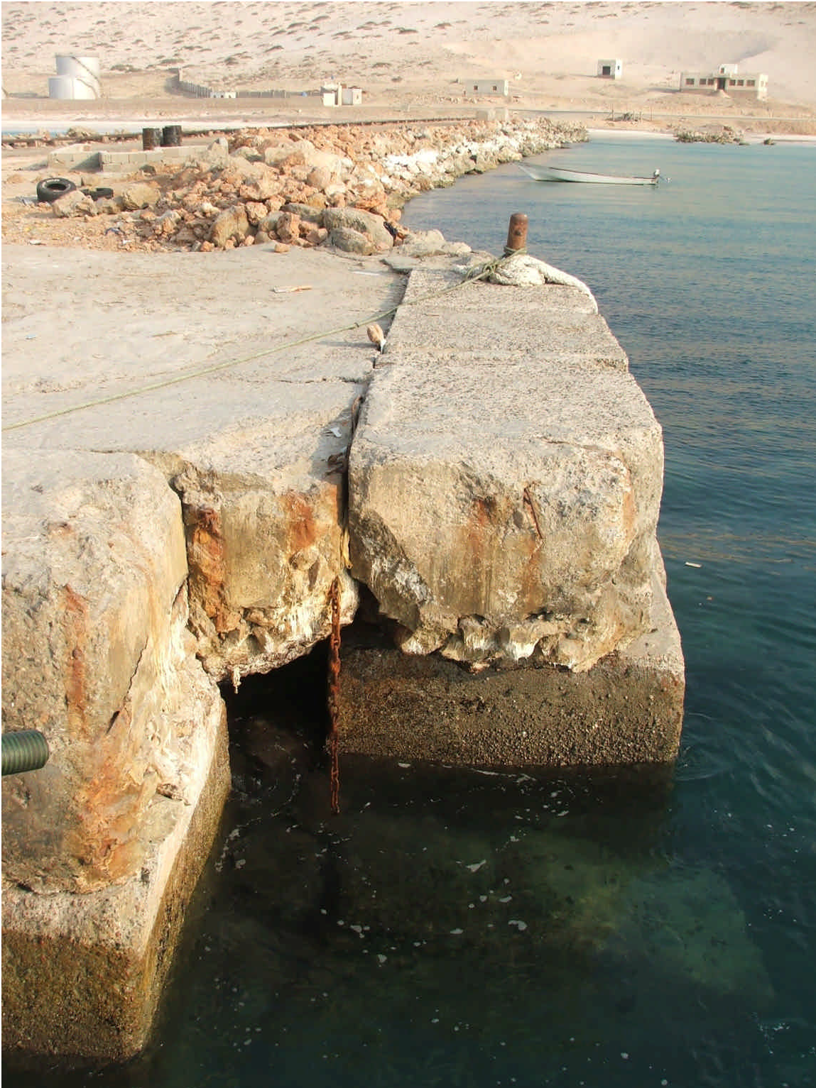
Figure 16 Damage to the loading stage with the western tip partially collapsed and corner stones fallen a sea, a petroleum storage facility and few isolated buildings in the background across the highway (view from berthed vessel).
