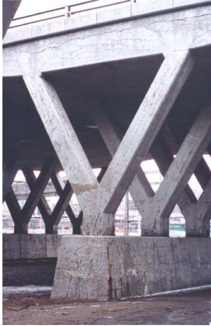
Figure 1.1. ASR in 20 year old highway bridge [1].
