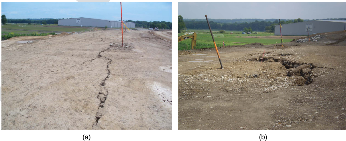
F3:1 Fig. 3. (a) Overview of top of compacted embankment in vicinity of slope failure prior to failure; and (b) close-up of scarp that developed on F3:2 embankment crest after slope movement.
