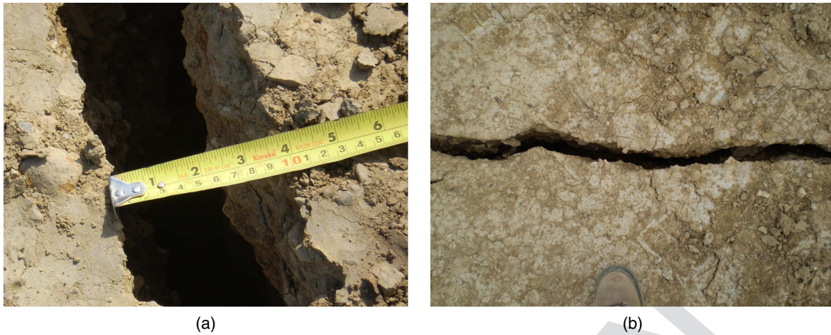
Fig. 4. Open tension cracks on top of compacted embankment in vicinity of slope failure at an embankment height of 2.4 m (8 ft).
