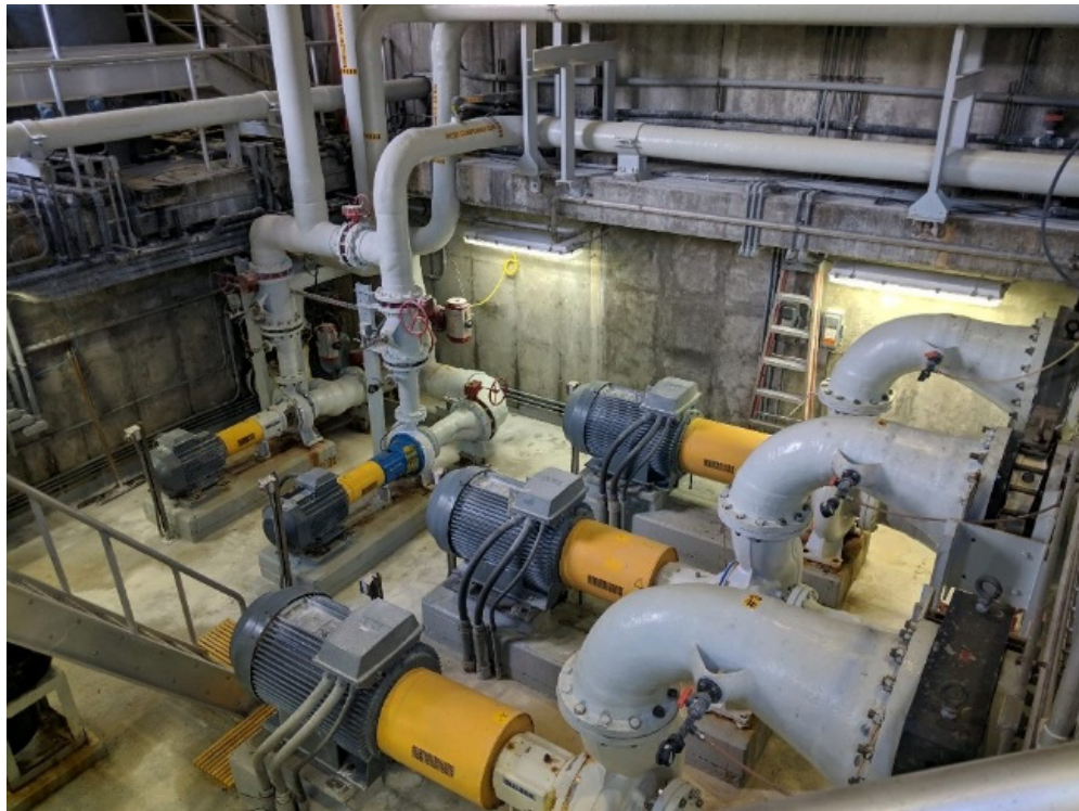
Figure 30: Tampa Bay Desalination unit pumps, courtesy of Tampa Bay Water.
