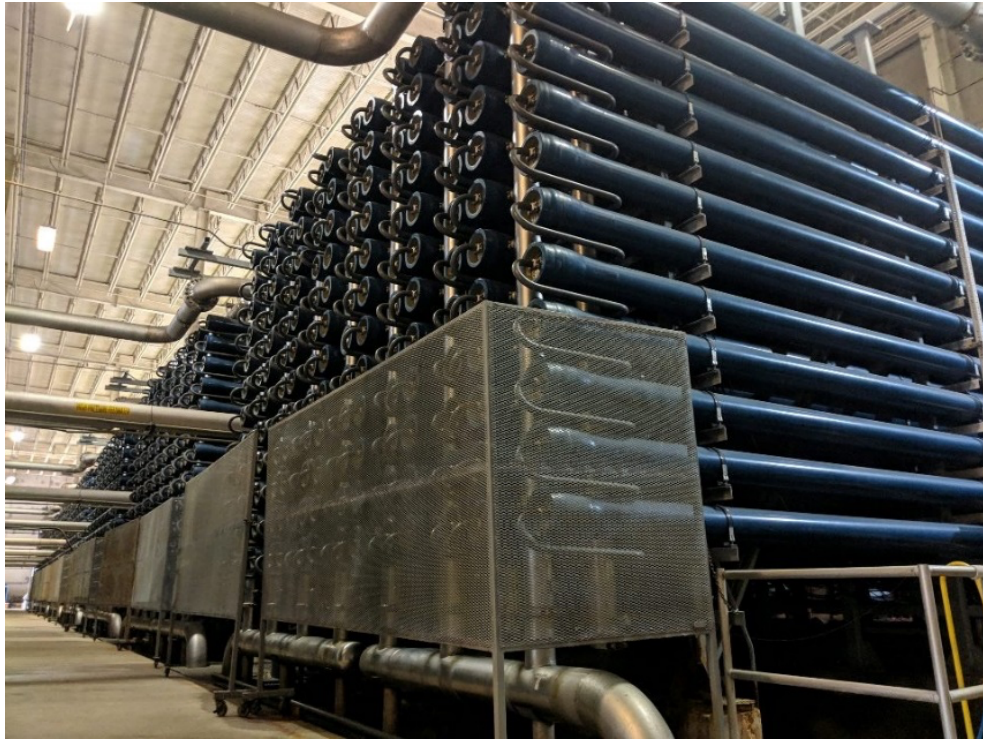
Figure 31: Tampa Bay Desalination plant reverse osmosis units.
