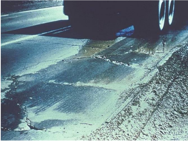
Figure 2-9: Water bleeding in concrete pavement (FHWA 2003).
