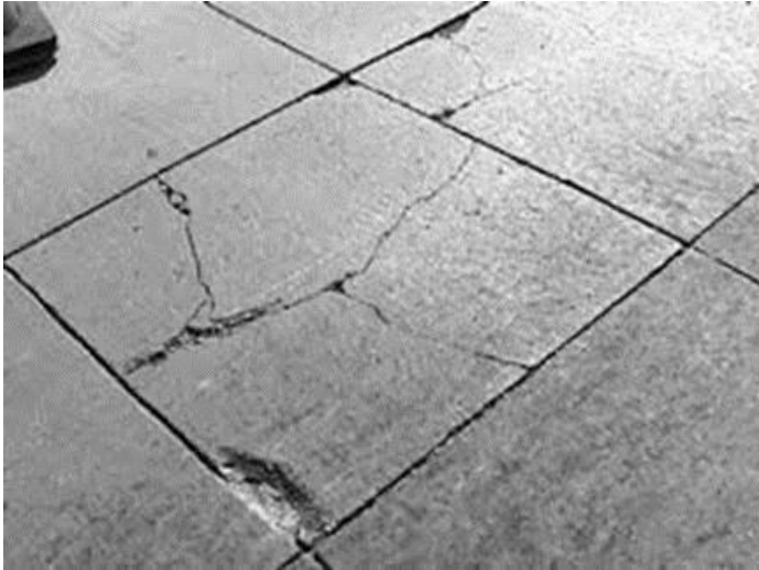
Figure 2-8: Shattered Slab ( The Constructor-Civil Engineering Home 2017 ).
