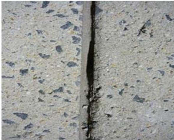
Figure 2-7: Medium level of joint seal damage (FHWA 2003).
