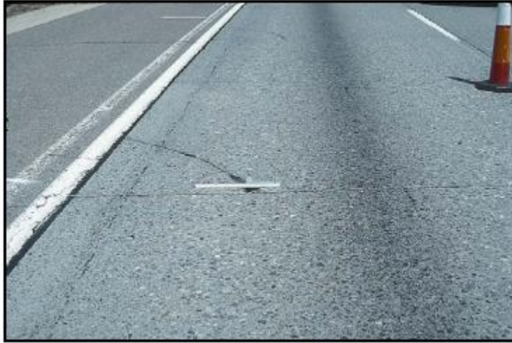
Figure 2-5: Corner Breaks in concrete pavement (FHWA 2003).
