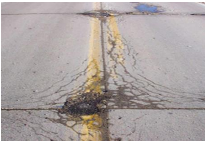
Figure 2-6: D-cracking in concrete pavement (Desta 2014).
