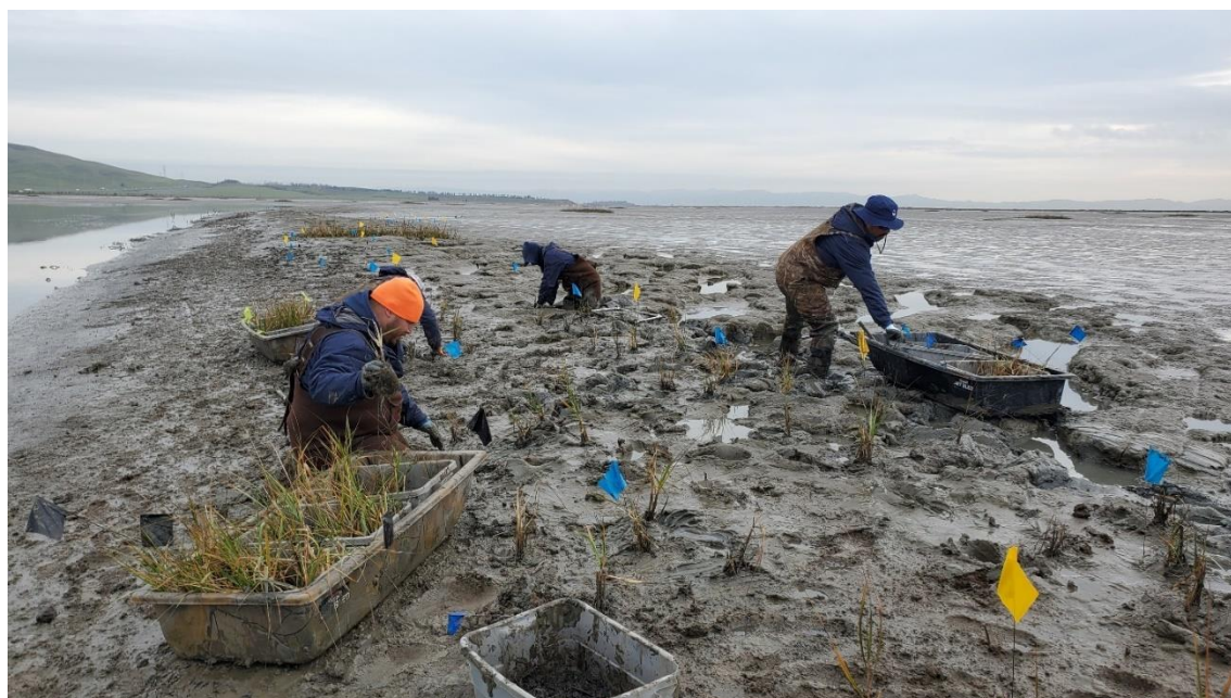
Figure 15: Adaptive management of raised earthen mounds to address wind driven erosion at the Sears Point wetland restoration, 2021. Pacific cordgrass is being planted to promote rapid vegetation spread over the earthen mounds within the site.
