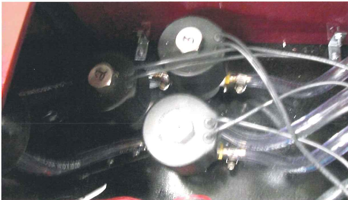
Figure 6: Solenoid Valves and Internal Fluid Lines
