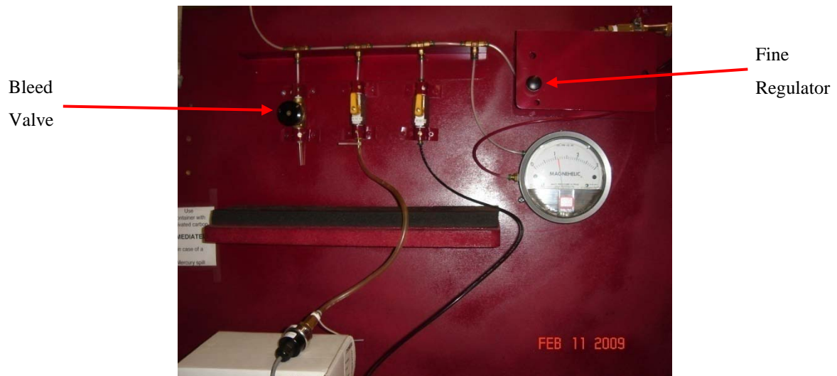
Figure 8. Fine and bleed valve pressure tuning
