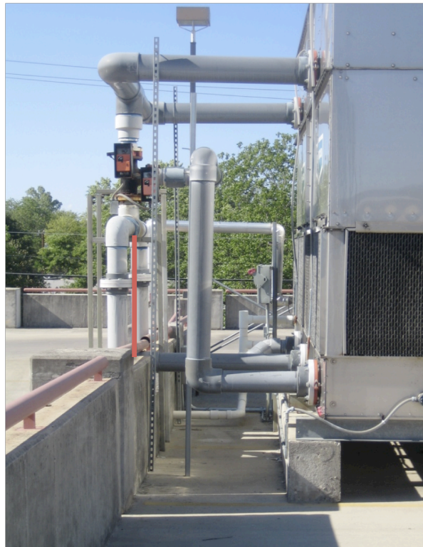
Figure F-5: Pipe Carrying Condensate Water at the Cooling Tower
