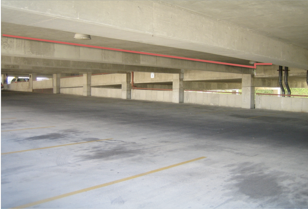
Figure F-4: Pipe Carrying Condensate Water to Cooling Tower, Location Second Floor of Parking Garage
