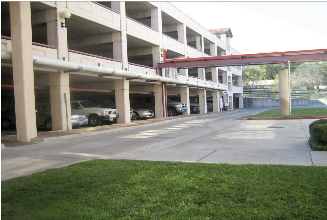
Figure F-3: Pipe Carrying Condensate Water to Cooling Tower
