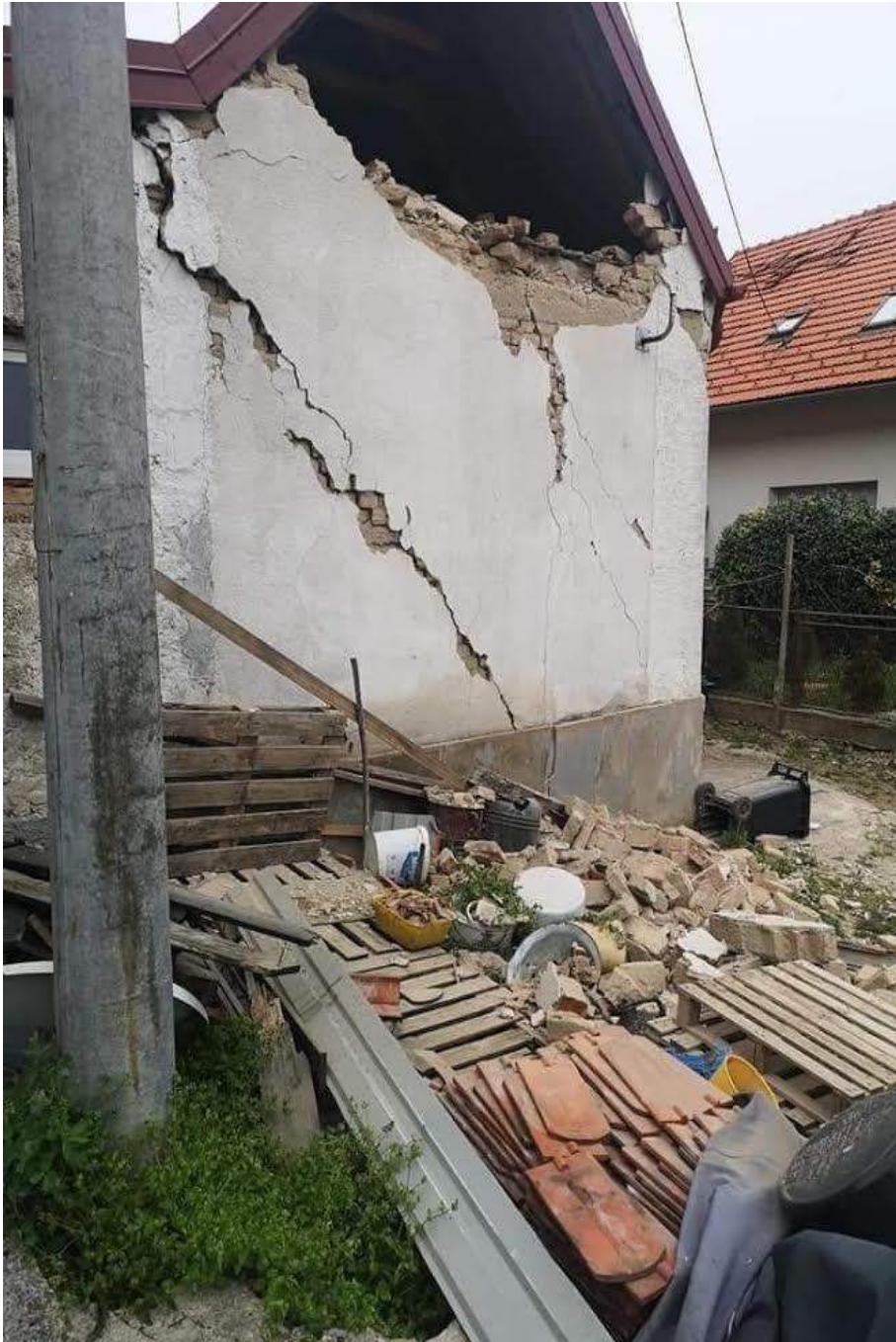
Figure 5-15 – Gable failure, credits to Dolores Rogic
