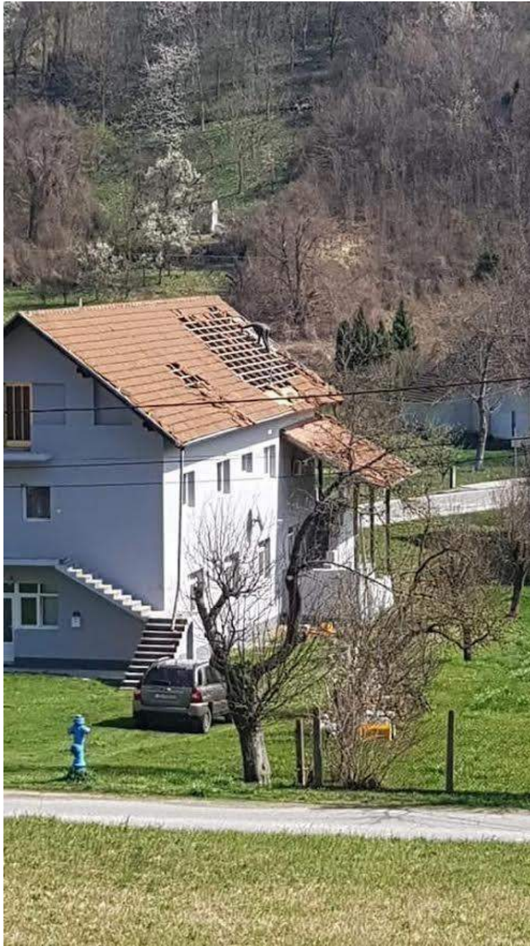
Figure 5-14 – Roof damage, credits to Dolores Rogic
