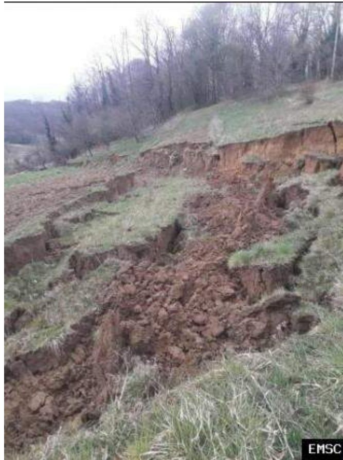
Figure 3-14 – Slope failure tagged as 6km from the epicentre on the EMSC website but not supported in any other official sources. https://www.emsc-csem.org/Earthquake/Gallery/?id=840695
