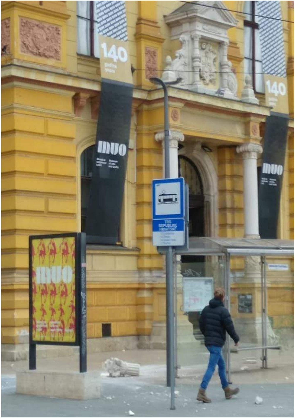
Figure 5-5 – Damage on the façade of the Museum of Arts and Crafts (MUO)
