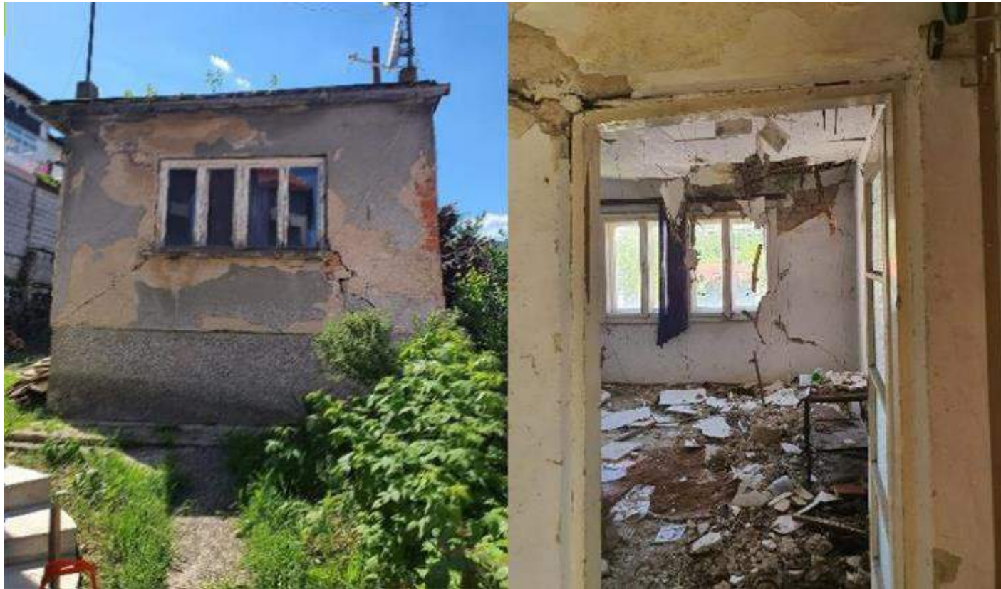
External and internal damage to a house in Orehovečki brijeg
