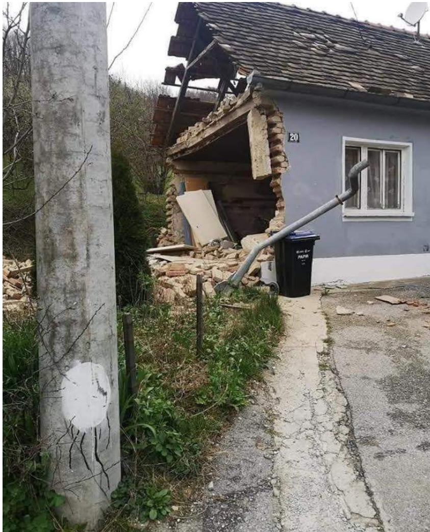
Figure 5-13 – Collapse of the whole façade – credits to Dolores Rogic
