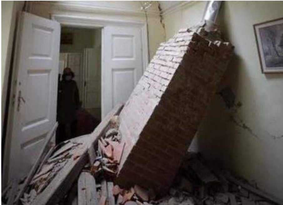
Figure 5-1 Damage of chimney falling indoor Source: City of Zagreb
