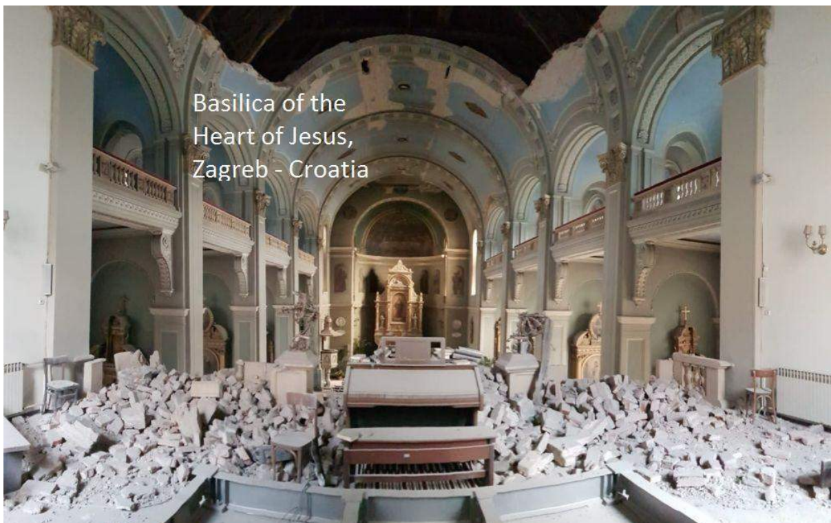
Figure 5-4 – Indoor damage of the Basilica of the Heart of Jesus – Zagreb
