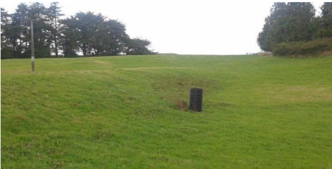
Figure 2.2: Photo of an upstand riser installed in the ponding area of a detention bund. The riser is connected to an outlet pipe that passes through the bund, which discharges ponded runoff on the downstream side.
