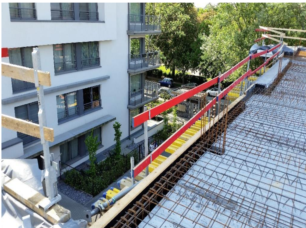
Picture 6.1.2-5 Safety issue noticed in Block 1 at beginning of the research (handrail missing, 4th floor)
