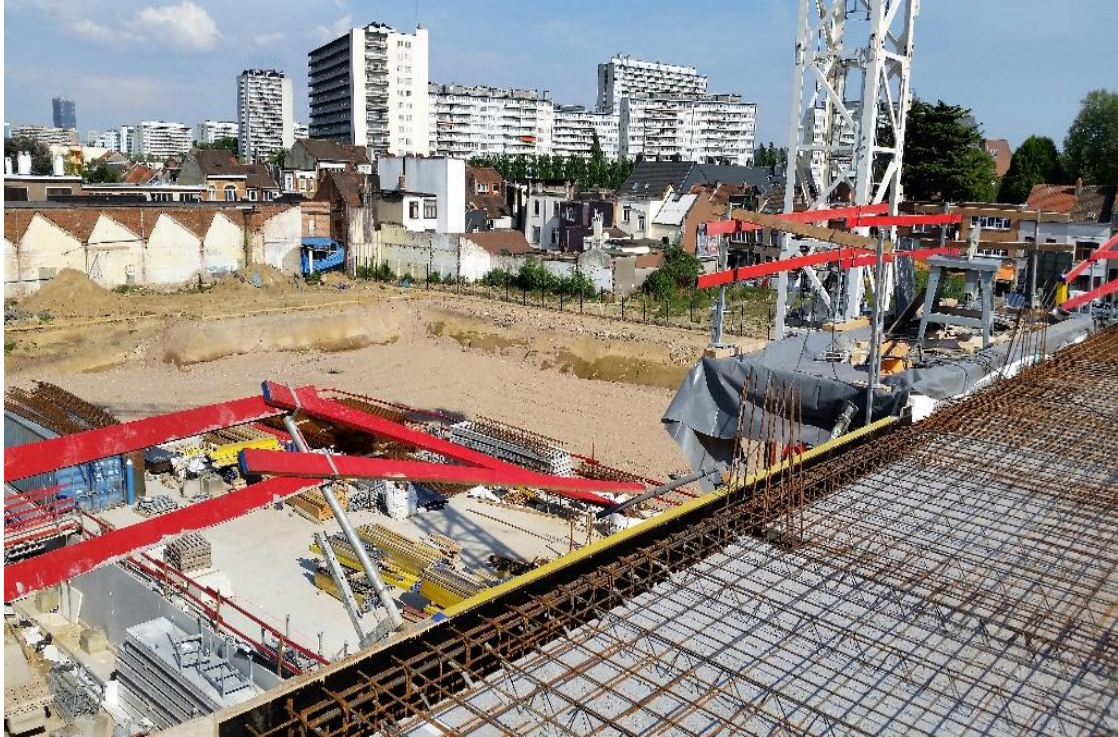
Picture 6.1.2-6 Safety issue noticed in Block 1 at beginning of the research (handrail missing), 4th floor
