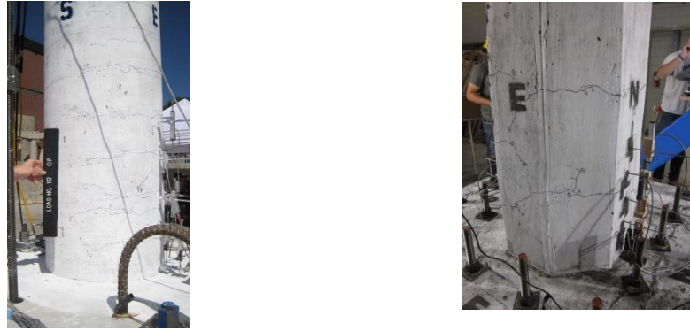
Figure 3. 3 Samples of RC Bridge Column Condition at DS-2 [45], [46]
