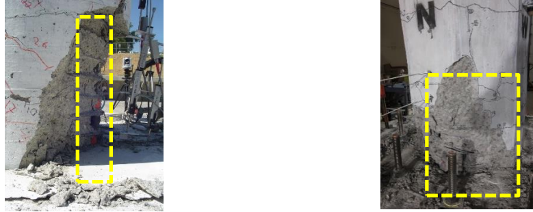
Figure 3. 6 Samples of RC Bridge Column Condition at DS-5 [45], [46]
