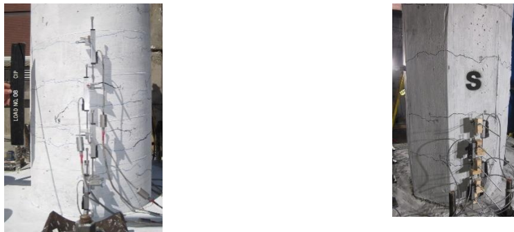
Figure 3. 2 Samples of RC Bridge Column Condition at DS-1 [45], [46]
