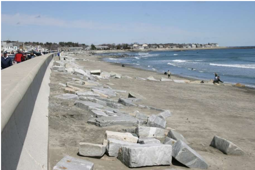
Figure NB-6. During storms, sand can be eroded from the lower beach and transported landward building a sand ramp against the seawall as seen here at North Beach on April 7, 2018 following three severe nor'easters. During this event, the sand extends from mid beach to the seawall.
