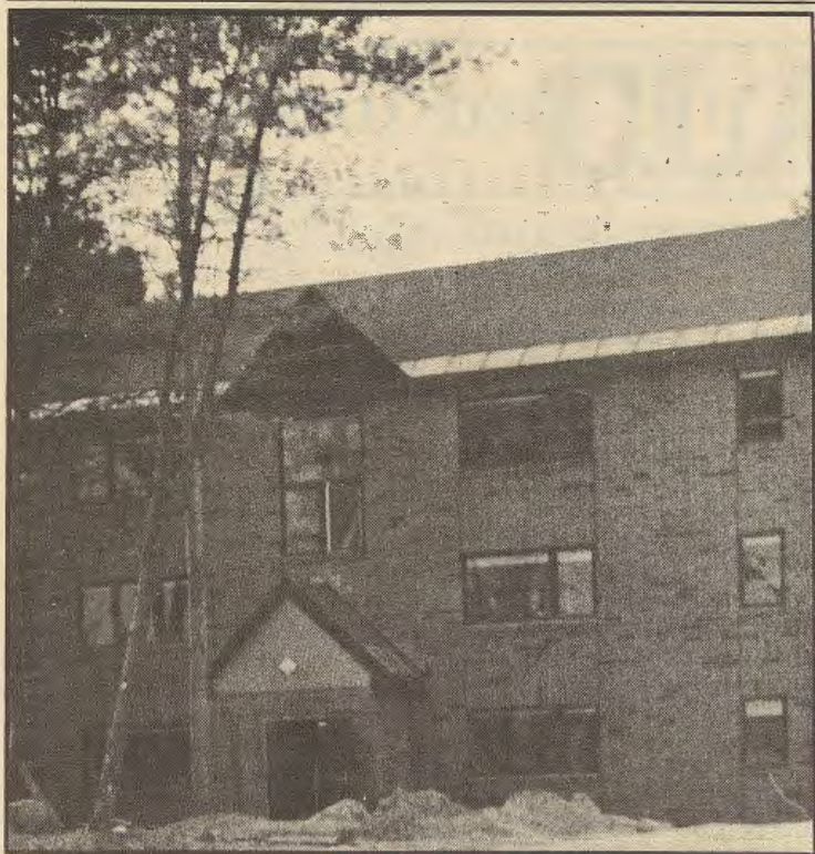
Work is being done to finish the remaining new dorms. (Rob Bossi photo)
