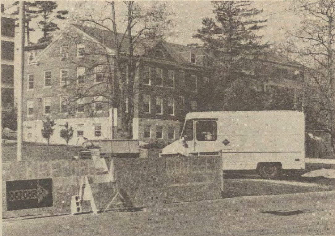
Vehicles pass over Nesmith lawn as construction of Area II heating system continues. (Tim Skeer photo)
