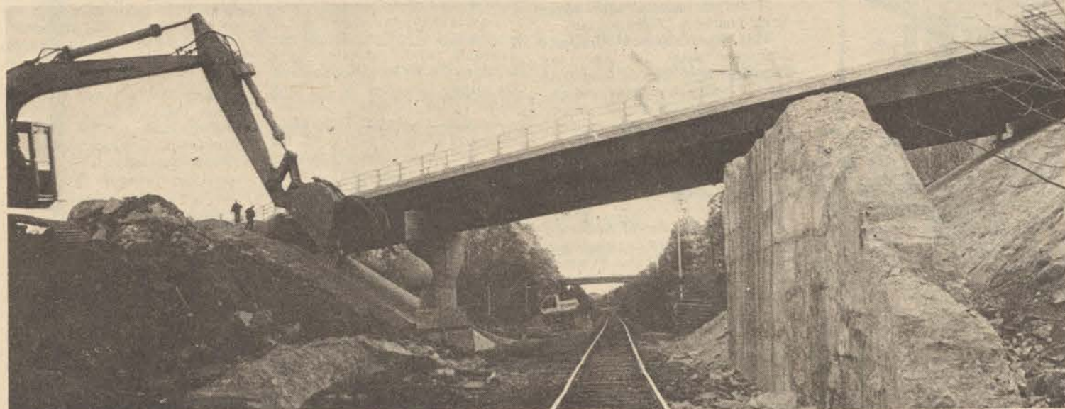
Traffic is now allowed on the new bridge on Madbury Road which leads from Durham to Dover. The bridge, financed by federal and state funds, replaces the old narrow, winding bridge and should be completed by the end of November. The new bridge is designed to be much safer to drive on and will hold more weight than the old bridge. (Barbie Walsh photo)
