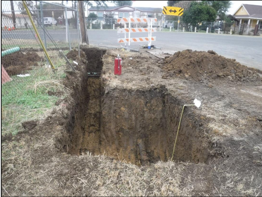
Figure 5-8. Overview of tie-in pit excavation and linear trench within the Leal Road ROW, facing northeast. Note the existing gas main on the right side of the pit, foreground, and the existing unknown utility within the linear trench, background.
