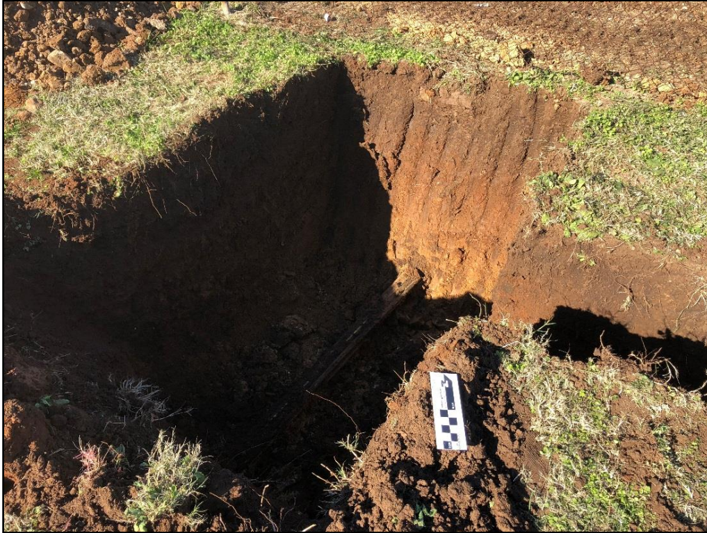
Figure 5-5. Bore exit pit along the southwestern side of Martinez Losoya Road, facing north.
