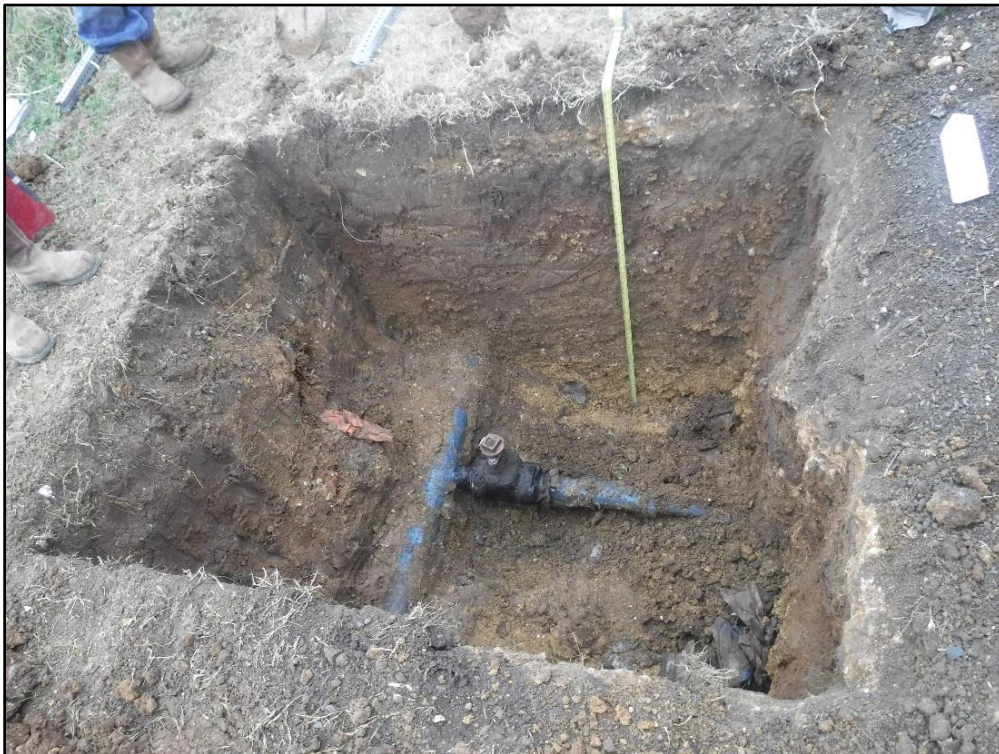
Figure 5-9. Example of "T" valve exposed to cut off the existing gas main for tie-in, facing north.
