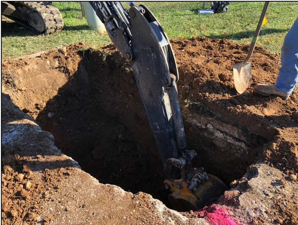
Figure 5-4. Bore entrance pit along the northeastern side of Martinez Losoya Road, facing west-northwest.
