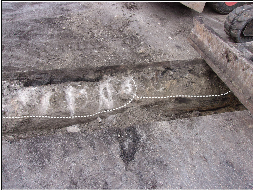
Figure 4-2. Trench profile depicting previous road layers and road base associated with multiple street modifications. Dotted white lines to the left show old concrete, to the right show layer of road base.
