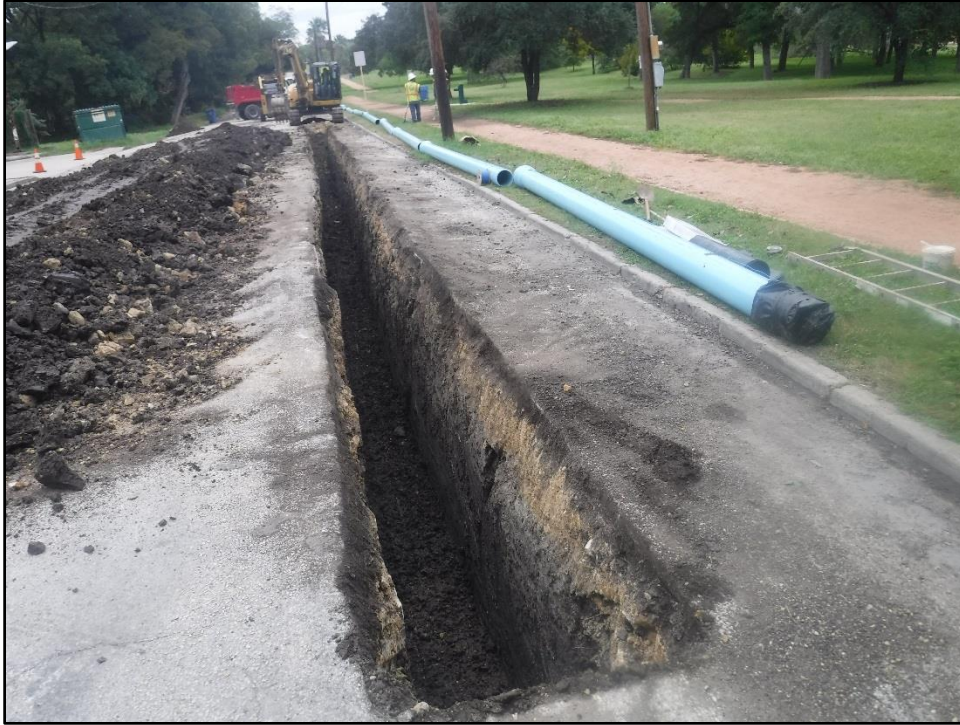
Figure 5-13. Overview of water main installation excavations along the southern boundary of the Parland Place ROW, facing east-southeast.
