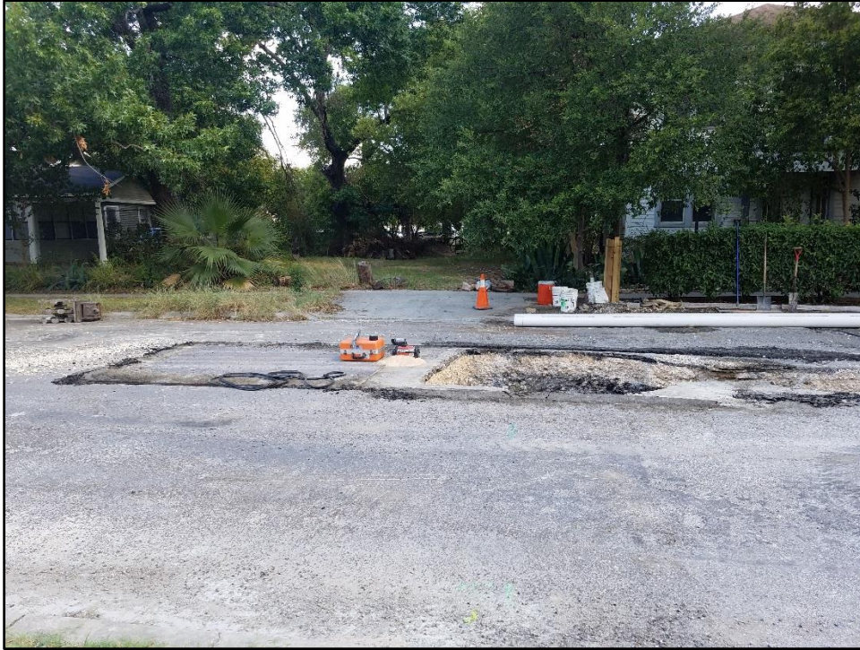
Figure 5-10. Overview of grassy ditch projection in relation to APE and new sewer main manhole installation, facing north.
