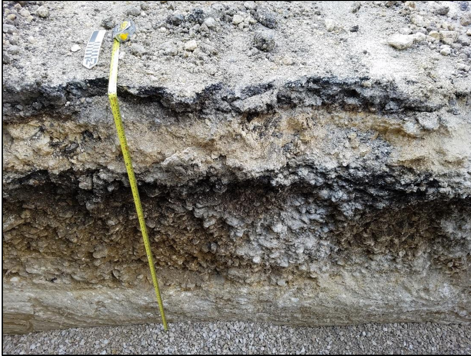
Figure 5-9. Average soil profile at the eastern end of the APE during sewer main installation excavations, facing south.
