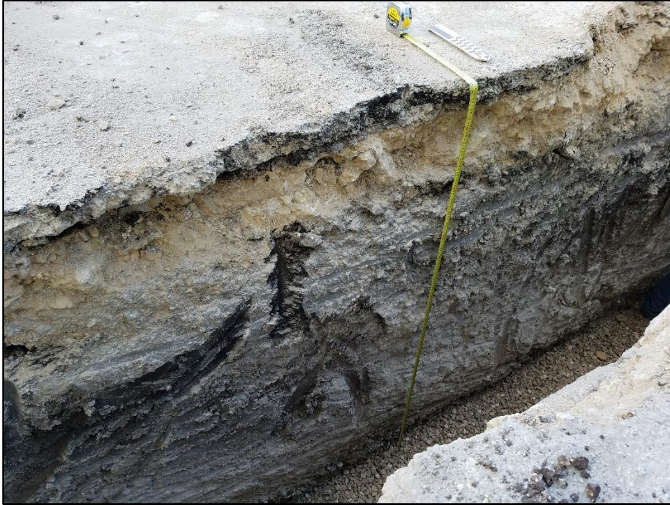
Figure 5-5. Average soil profile at the western end of the APE during sewer main installation excavations, facing southwest.
