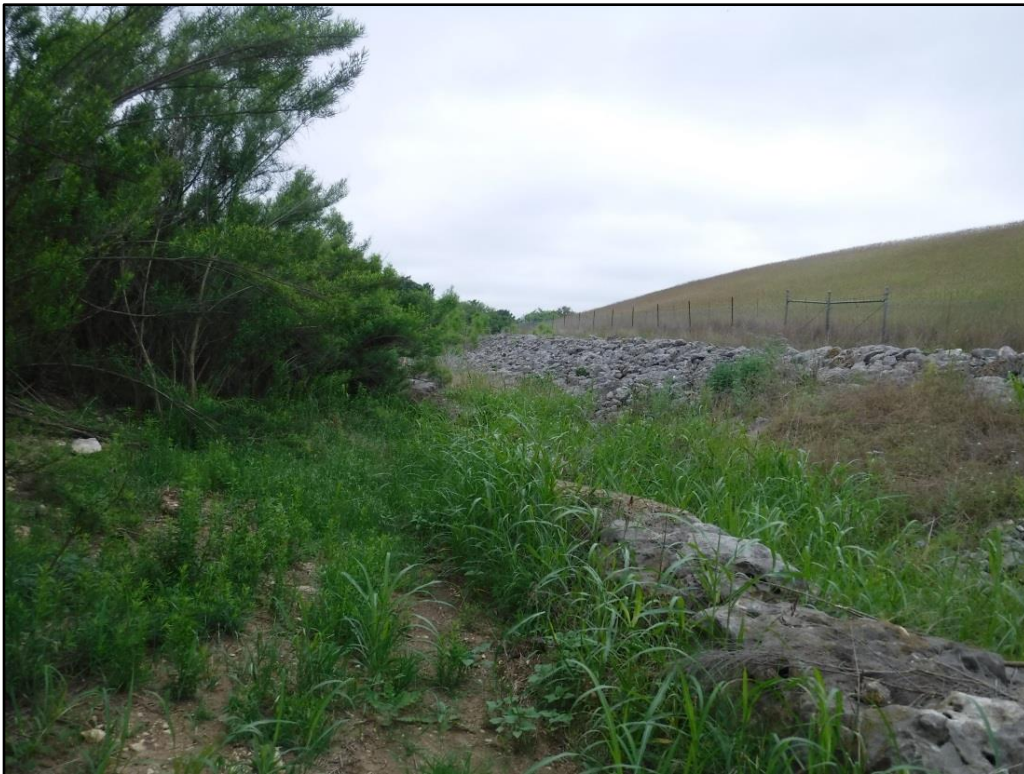
Figure 5-9. Overview of temporary access road that skirts the earthen damn within the golf course.
