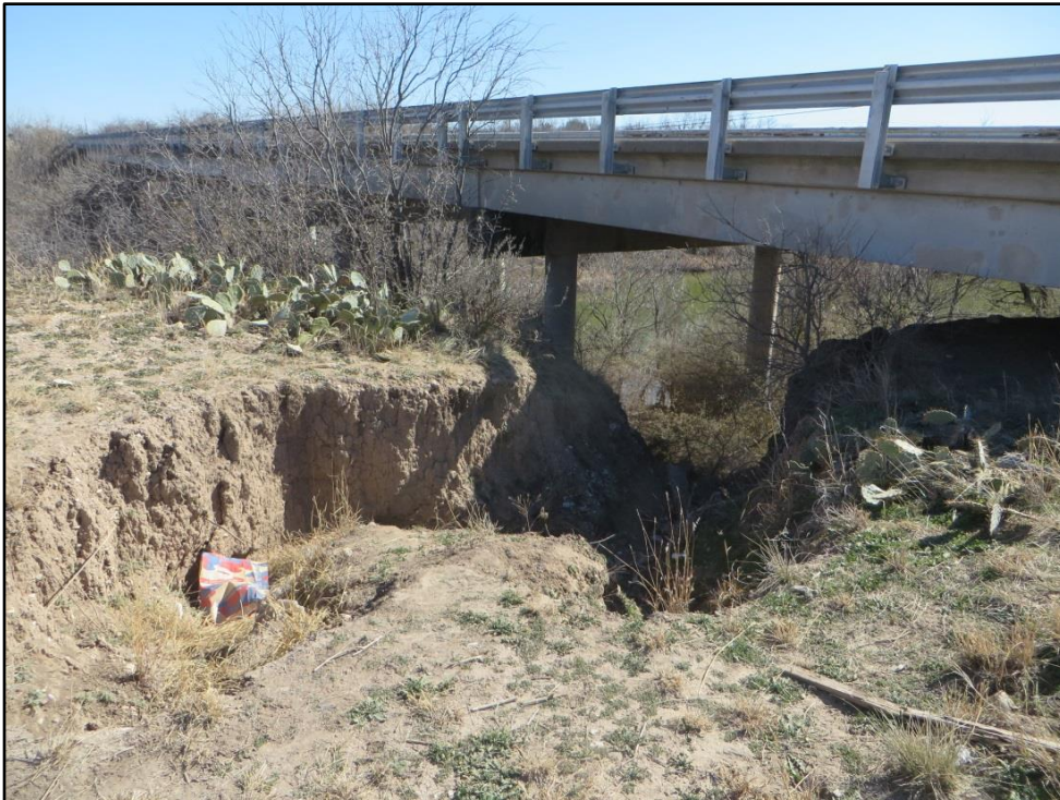
Figure 6-9. Erosional cut adjacent to ST6, facing southeast.
