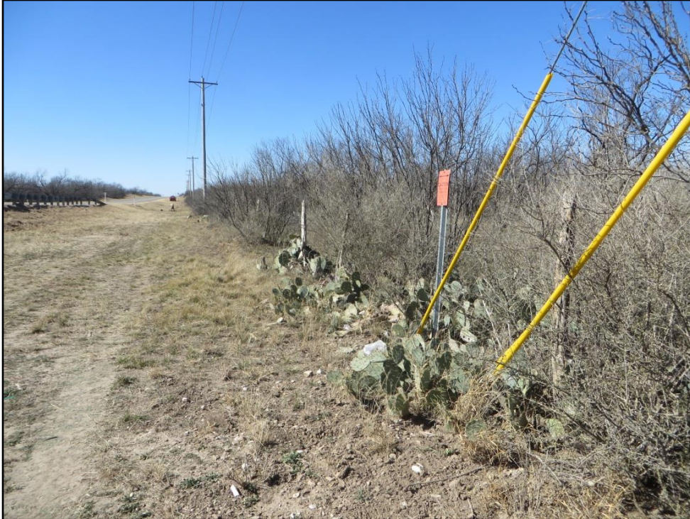
Figure 6-7. Overview of buried electric cable paralleling the fence line, marked with orange signage, facing west.
