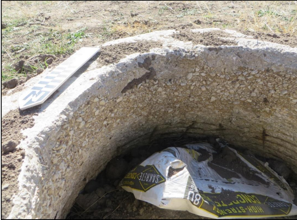
Figure 6-6. Close up of concrete matrix and hog-wire mesh framing of abandoned utility.
