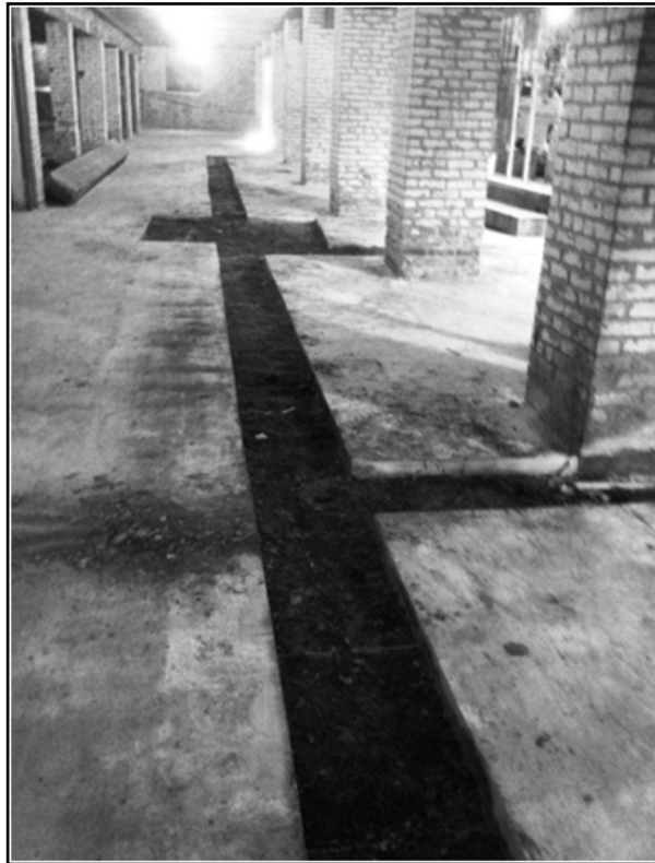
Figure 7-5. Photo of cut in basement floor of Building 1. View is to the east, toward the area of sump (see Figure 7-4). Photo courtesy of Kay Hindes, Office of Historic Preservation, City of San Antonio.
