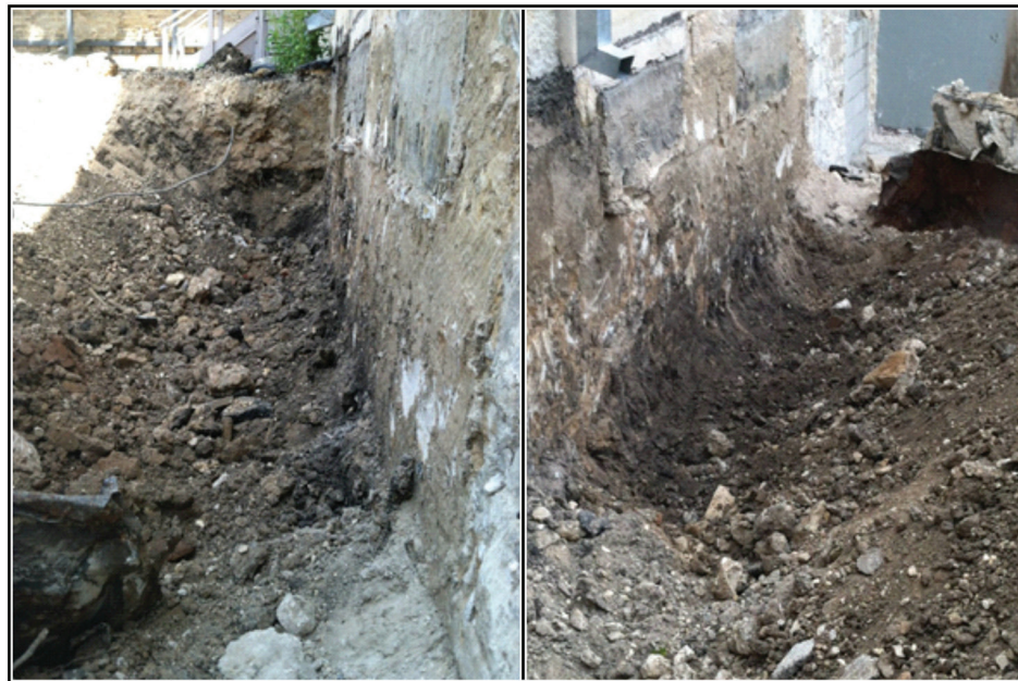
Figure 7-2. Photos of Trench 1, looking north (left) and south (right). Note dark soil at trench base and wall repairs.
