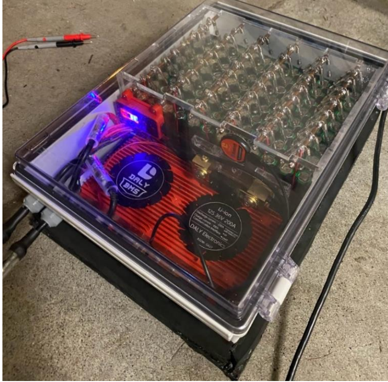
Figure 28: Lithium-ion Battery Box and System
