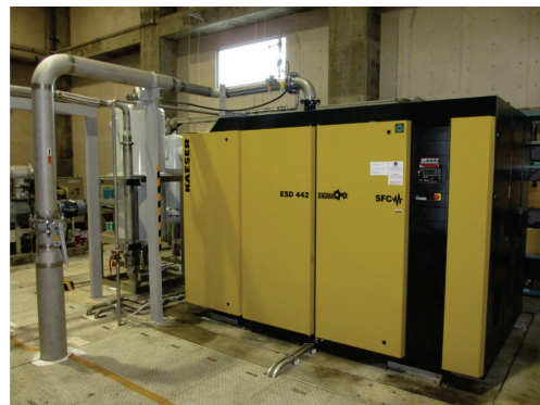
Fig. 1. Photograph of the new main compressor. The oil removal system is installed beyond the compressor.
