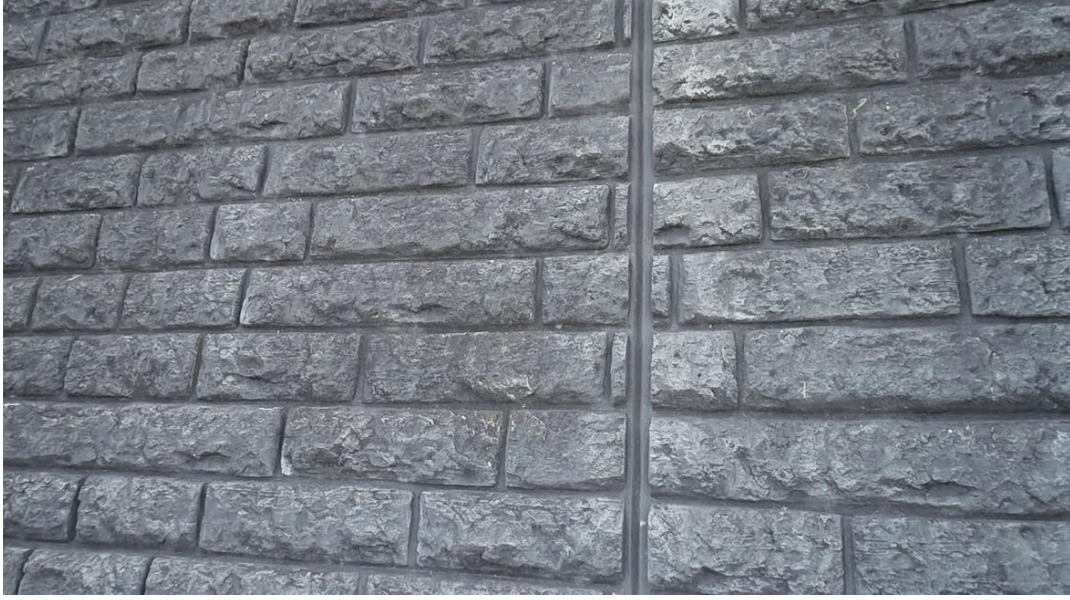
Figure 4.6: Concrete Block elements of the wall with significant obvious weathering effect
