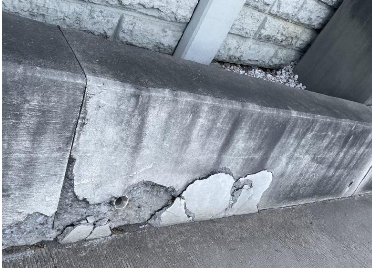
Figure 4.2: Concrete spalling observed on the base of the wall
