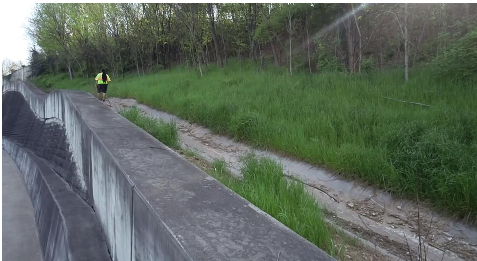
Figure 4.5: Drainage channel at the top of the wall clearly defined, albeit with little to no blockage
