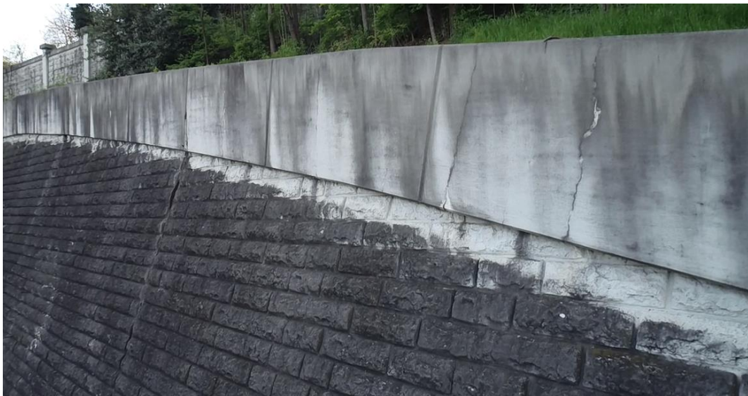
Figure 4.7: Noticeable presence of efflorescence and moderate-to-wide cracks
