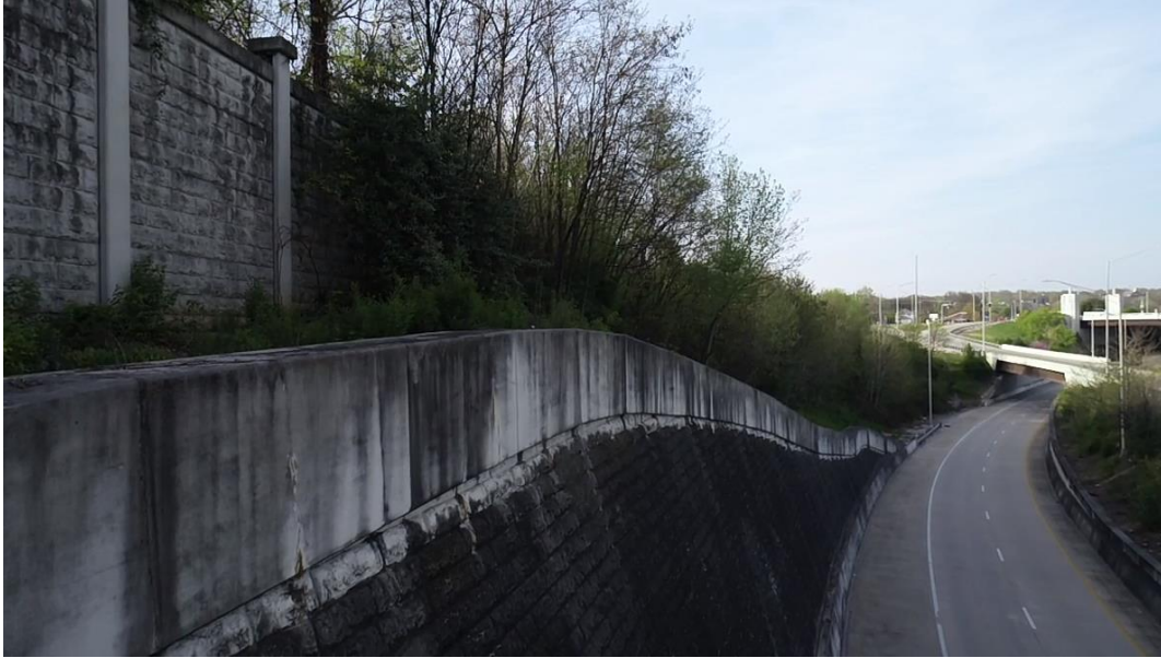
Figure 4.8: Aerial view of wall showing adjoining traffic and no traffic barrier
