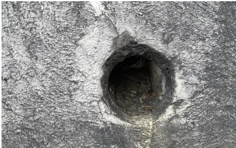
Figure 4.3: Drain at the base of the wall partially clogged
