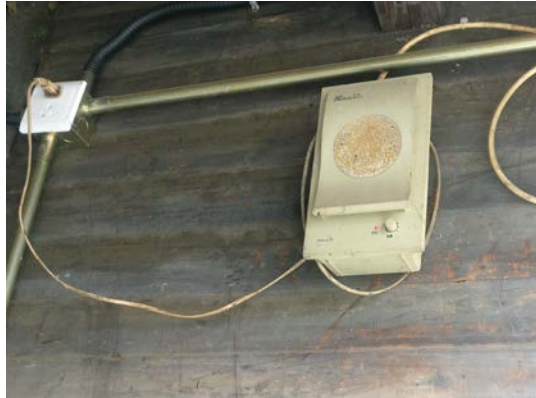
Figure 2 Example of a small loudspeaker that is still functioning
