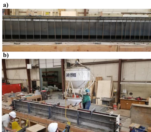
Figure 4.5. View of the (a) beam reinforcement before casting and (b) beam during construction
