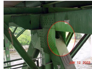
(c) Buckled gusset plates - National Transportation Safety Board
