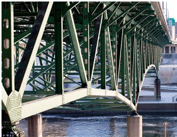
(a) Before collapse - Side view of the bridge showing steel structural members
