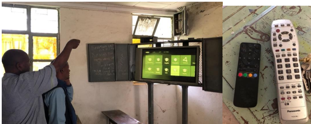
Figure 6.14 Normal Plasma system and the remote in the next classroom in Bole
