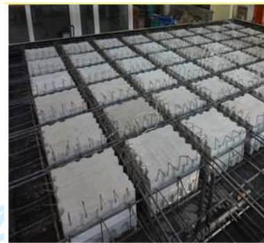
(k) Layout of exposed assembly boxes
