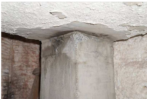
(g) South-east corner column in Test 2
