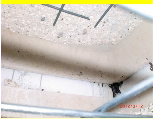
(e) Spalling on the top plate of the assembly box
