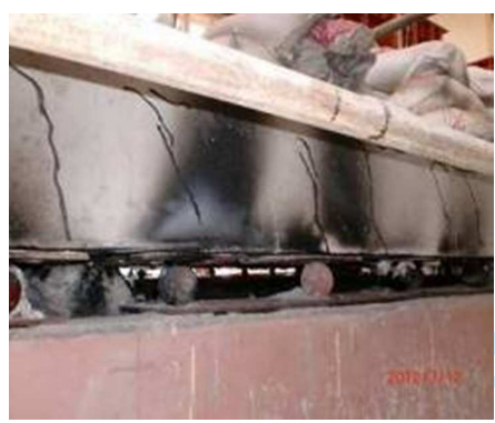
(c) Inclined cracks on the edge beam
