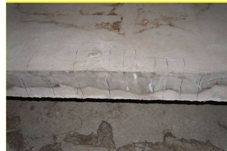
(f) Edge beam in Test 2
