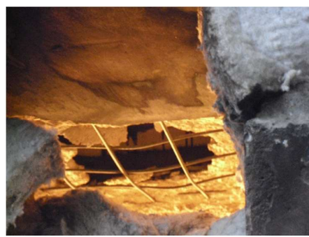
(b) Spalling of assembly box
