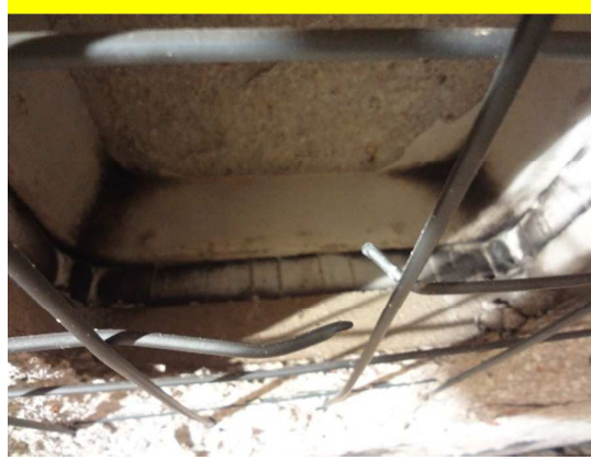
(e) Steel fracture and spalling of the assembly box
