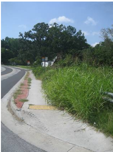
Figure 2.2-10: Some of the sidewalks in the study area lack adequate maintenance.
