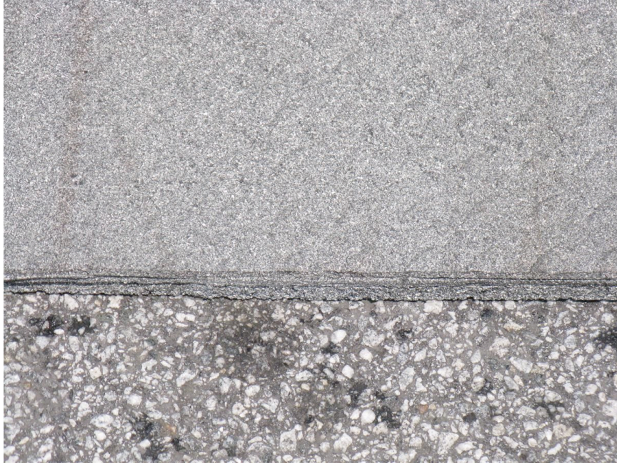
Figure 52 – Close-Up of Detector Pad, Showing “Fleck” Paint Blending with Pavement
