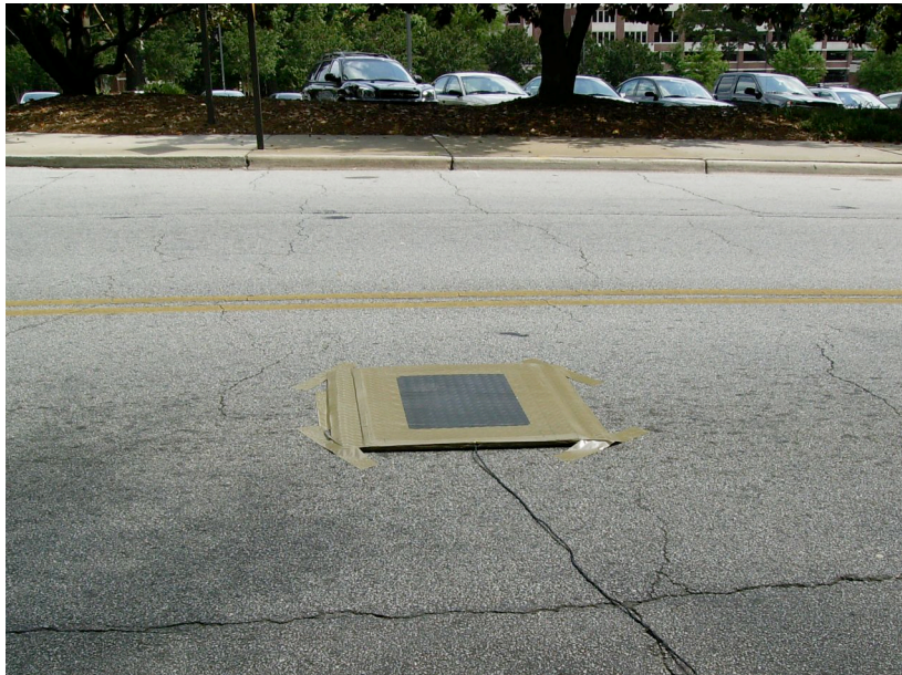
Figure 17 – First Generation Loop Pad (17" X 34" Loop) Affixed to Eastbound Ferst Drive on Georgia Tech Campus
