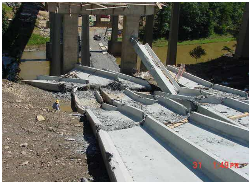
Figure 1.2 - Stability failure of precast prestressed concrete girders on I-80 in Pennsylvania (Zureick, Kahn and Will, 2005)
