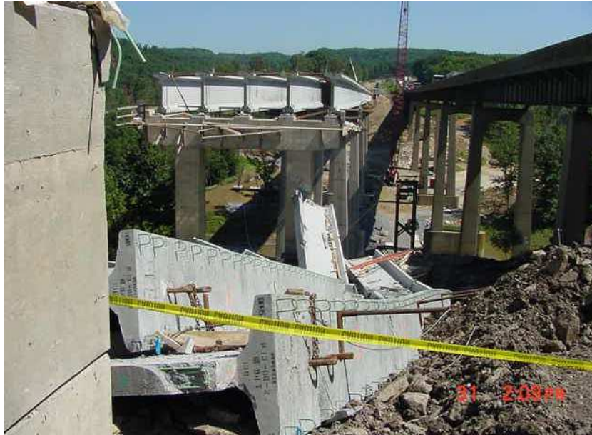
Figure 1.1 - Stability failure of 90 in. (2.3 m) deep precast prestressed concrete girders on I-80 in Pennsylvania (Zureick, Kahn and Will, 2005)
