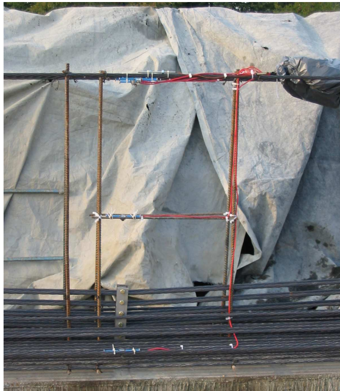
Figure 3.5 – Internal vibrating wire strain gages and thermocouples
