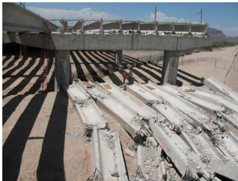
Figure 1.3 – Stability failure of AASHTO Type V bridge girders in Arizona (Oesterle et al., 2007)
