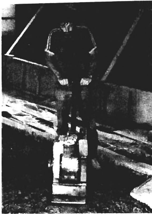
FIGURE 36. JAY-12 VIBRATING PLATE COMPACTOR USED TO OBTAIN 100% OF T-180 DENSITY IN CRUSHED STONE BASE.
