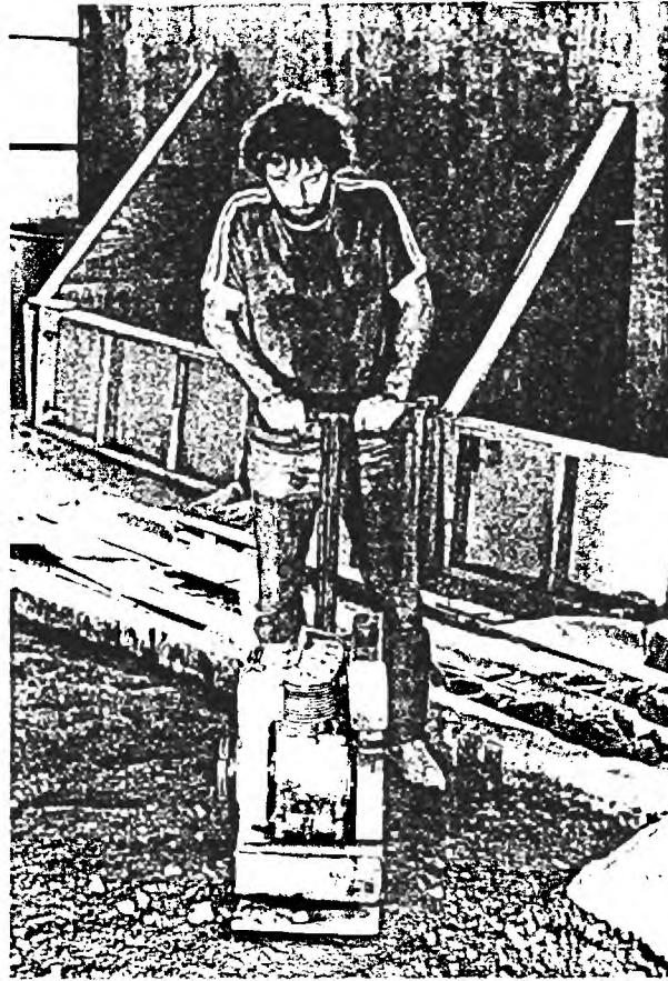
FIGURE 39. JAY-12 VIBRATING PLATE COMPACTOR USED TO OBTAIN 100% OF T-180 DENSITY IN CRUSHED STONE BASE.
