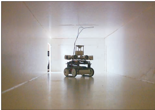
Figure 6. Deployment in an air duct.
