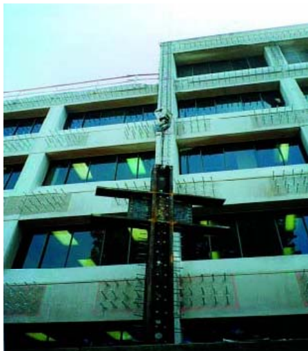
Figure 1.2: Seismic retrofit of the Administration Building, San Francisco State University, installation of prefabricated column-joint assembly [Kouyoumdjian, 1999]
