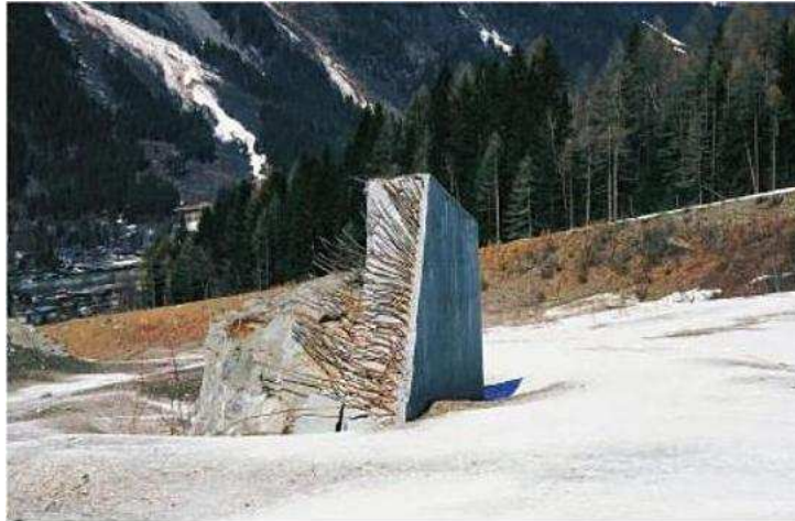
FIGURE 2. Protecting wall in armed concrete at Taconnaz (Haute-Savoie, France) destroyed by the powder-snow avalanche of the 11 February 1999. The height is 7 m and the thickness is 1.5 m (Photo by C. Ancey).
