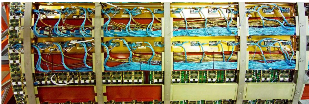
Figure 20. Partially assembled End Cap showing two full cable trays at the top and one empty cable tray at the bottom. Each tray carries cables for 1/32nd of the detector and acts as part of the outer Faraday cage of the detector. The blue cables are the 36 AWG data and control shielded twisted pairs, the heavier orange-brown cables are low-voltage supply cables. The light colored HV cables are just barely visible in the upper tray on the left. In this view the Triplet Boards serving the A type Wheel nearest the interaction point are on the left and the PPF1 connectors are just out of the picture on the right.
