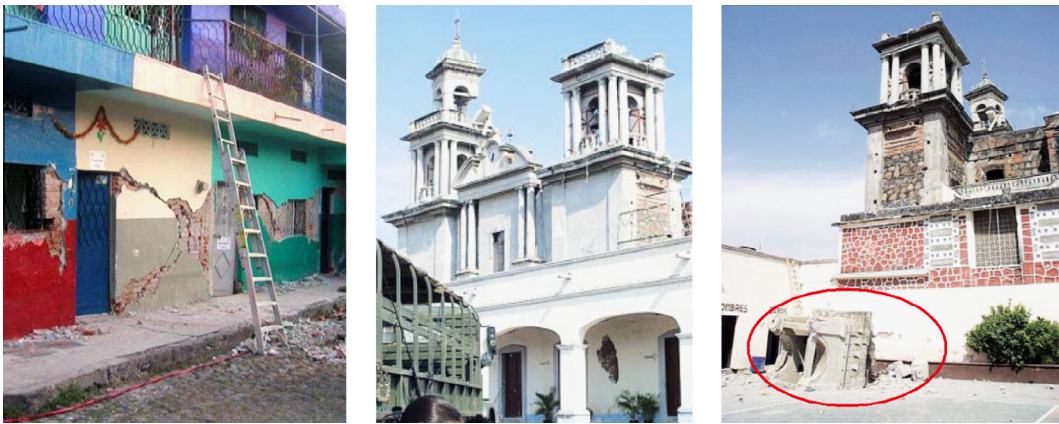
Fig. 2. Observed damages on churches after the 2003 M7.5 Colima, Mexico EQ.
