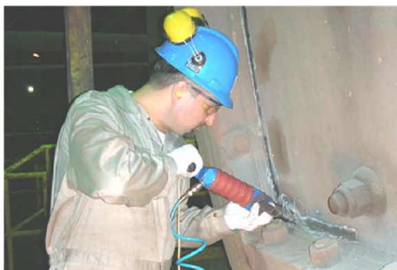
Fig. 13. Application of UP for rehabilitation of welded elements of a large grinding mill shown in Fig. 12
