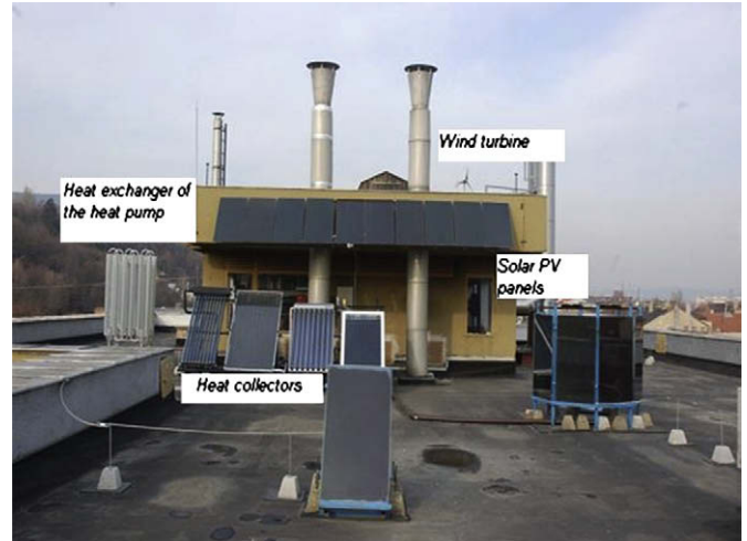
Fig. 1. Budapest Tech renewable system.
