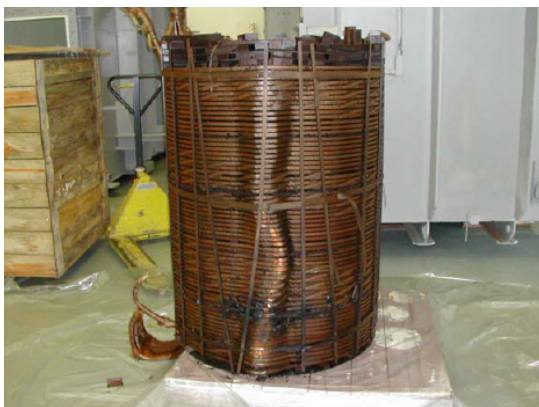
Fig. 4. Coil 1 damaged in the medium voltage winding.
