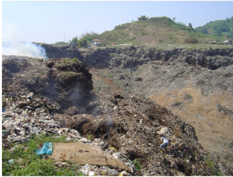
Figure 4 Scarp of the dumpsite after the February 2005 disaster. In the foreground, a scavenger carrying reusable material from the dumpsite. In the background, the steep natural slope in brown color (photo: F. Lavigne, July 2005).
