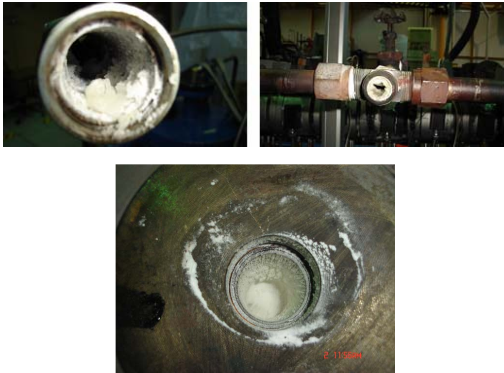
Figure 7.7: Pictures of vent lines clogged with product
