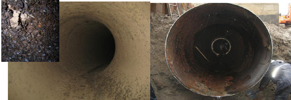
Fig. 1. Deterioration State of Medium and Large Diameter Steel Pipe of K-water.
