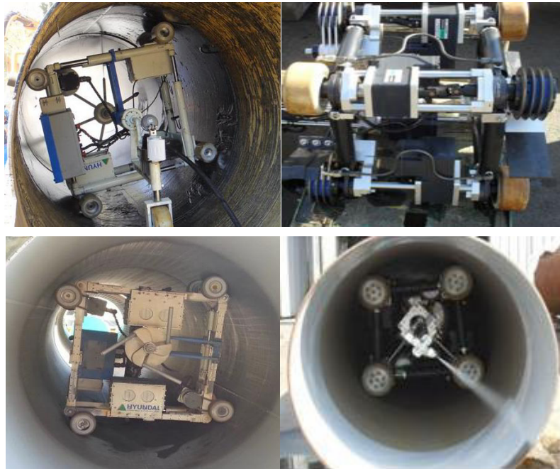
Fig. 3. SCSL Units: (top) High Water Pressure Jet Unit. Existing Coating Layer Scraping Unit; (bottom left); (bottom right) Spraying-on Lining Unit.
